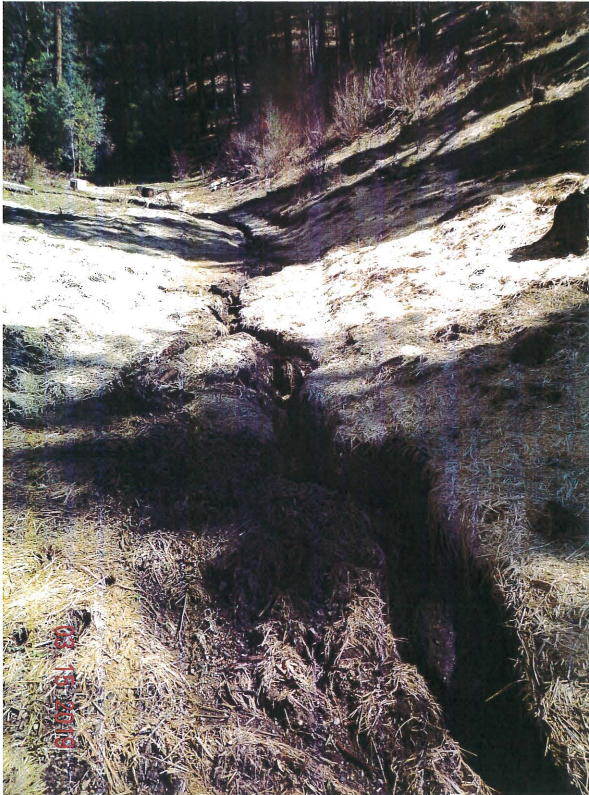
Figure 2. Unnamed stream tributary to Salt Creek where alteration, sediment and nutrient discharges, and trash were documented. Approximately 275 feet of the stream was graded and altered.
