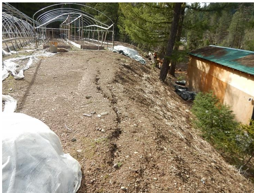
Photo looking south along western edge of GH1. Note tension cracks suggesting fill is unstable.
