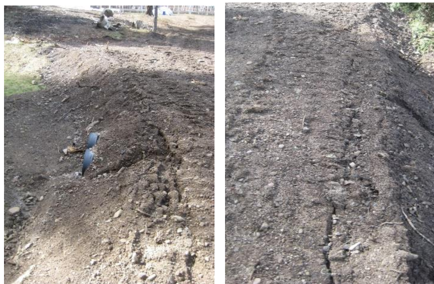
Pictures of north (downstream) and south (upstream) sides of newly constructed crossing (looking east). Note tension cracks near buttress tops and rills on both upstream and downstream slope faces suggesting crossing is susceptible to failure.
