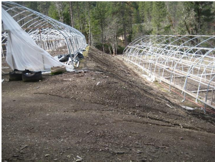
Eastern side of GH2 flats looking west. Note fill in middle of image.
