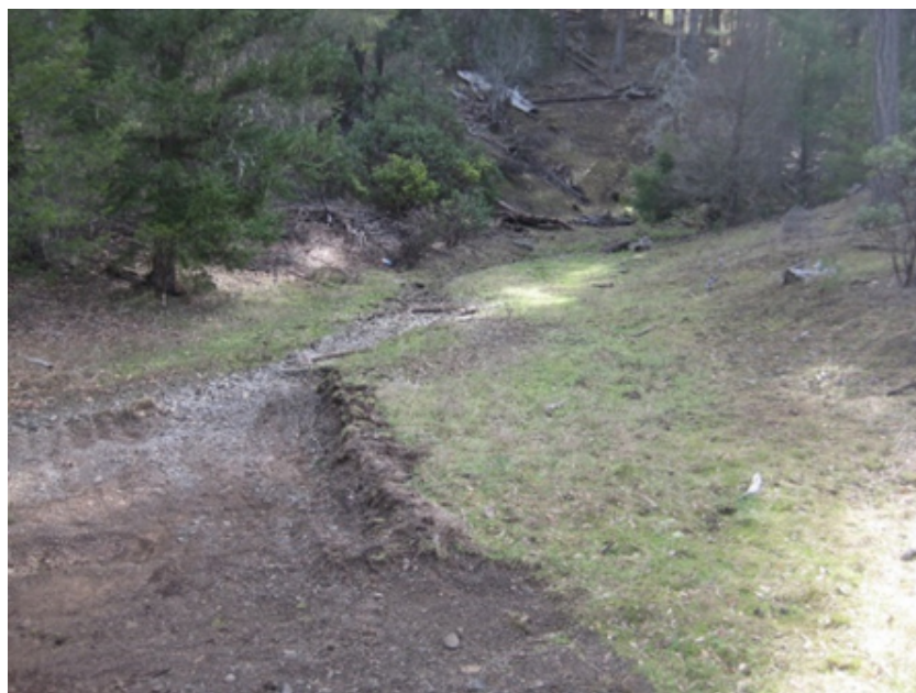
Channel upstream from newly constructed crossing (looking south). Note grading has removed vegetated floodplain and altered channel. Upstream channel width of five feet suggests the two 18-inch diameter culverts are too small to accommodate the natural flow regime.
