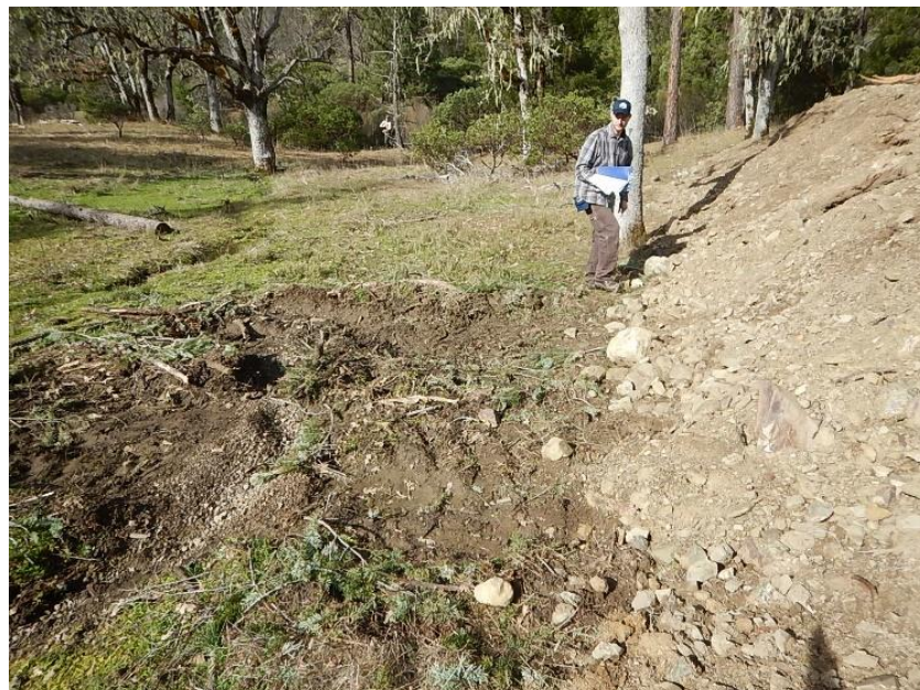
Pond southwest buttress encroaching on area with wetland indicators (looking northwest).
