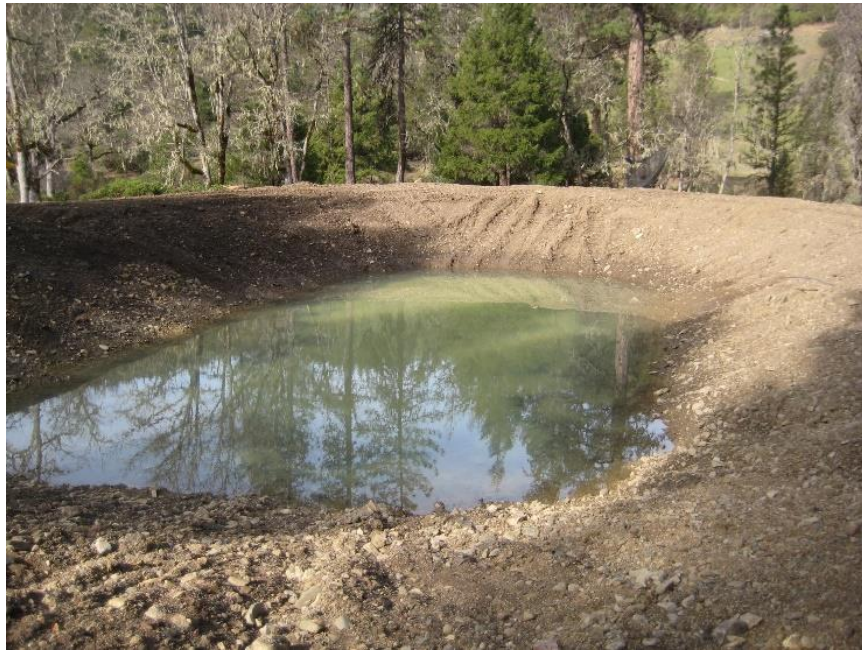
Newly constructed pond (looking northwest). The South Fork Mad River flows from left to right in the background of this image and its tributary passes along the left berm.
