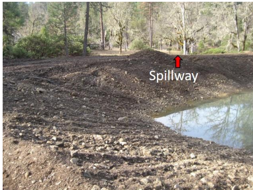
Newly constructed pond (looking southwest). Note berm on top of pond where earthen material was excavated for a spillway.
