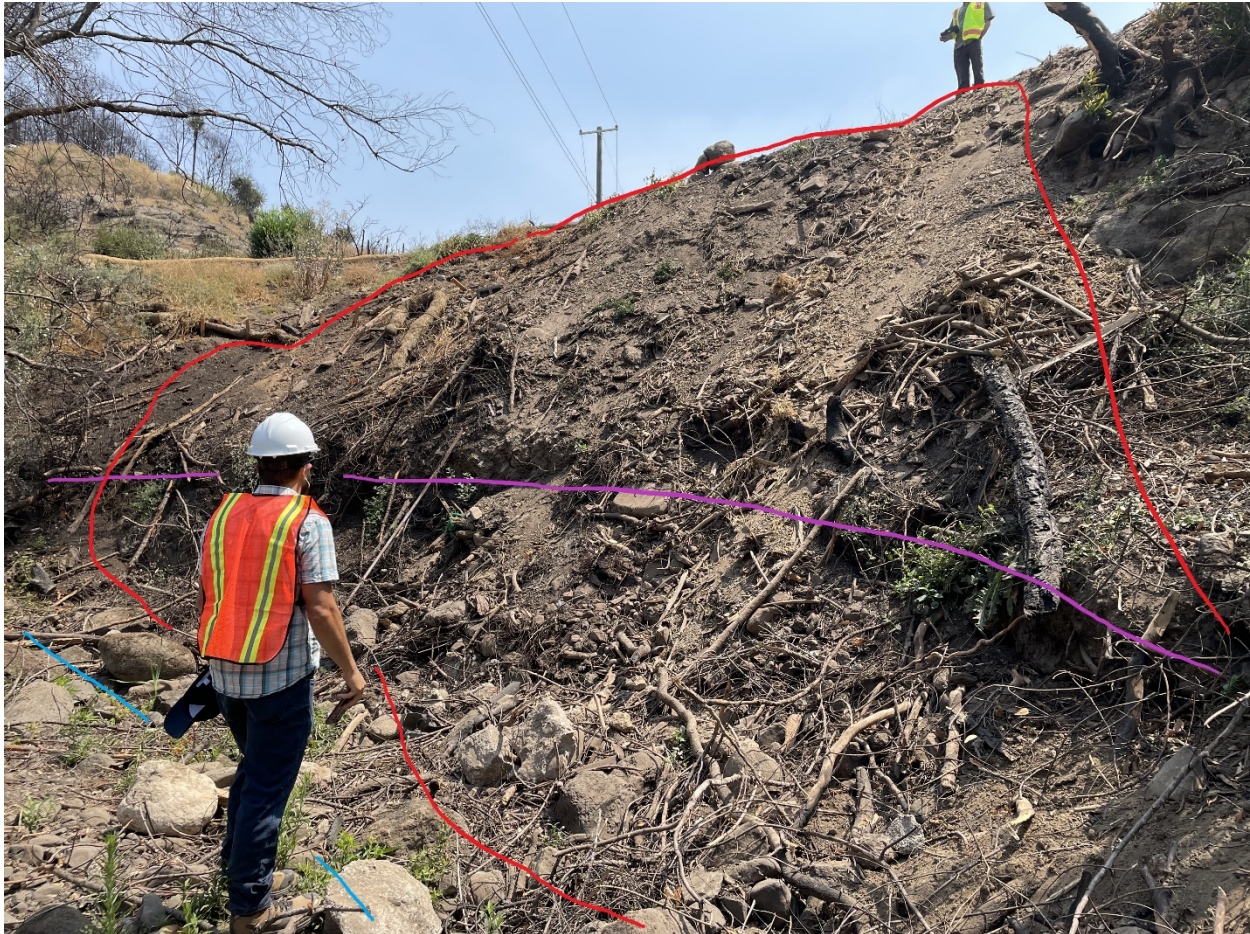
Figure 1. View of discharge from within channel of unnamed tributary. Red line: approximate extent of discharge. Purple line: approximate bankfull. Blue line: Approximate path of side channel during higher flows.
