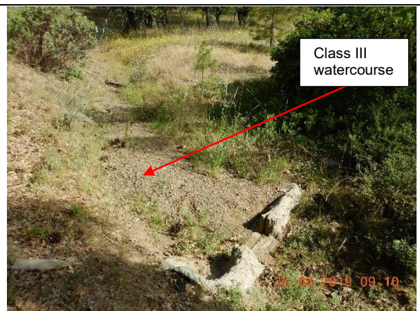
Photo Taken by: Pansy Yuen, 26 June 2019 Photo 12 – North view of an unnamed Class III watercourse with a concrete diversion structure installed across the width of the watercourse.
