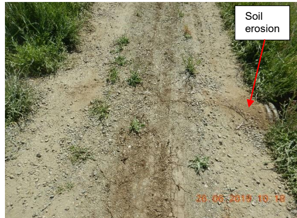
Photo Taken by: Pansy Yuen, 26 June 2019 Photo 56 – Top view of a second culvert under a main access road. Soil is eroding on top of a culvert inlet point. Evidence of erosion is shown in Photos 57 to 59.
