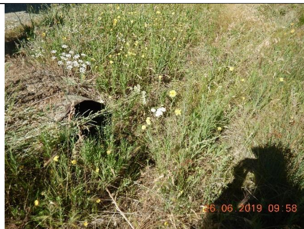
Photo Taken by: Pansy Yuen, 26 June 2019 Photo 54 – Southwest view of a culvert on the north side of a main access road downstream from the Class III watercourse.
