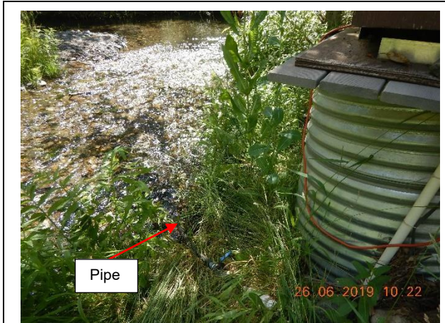
Photo Taken by: Pansy Yuen, 26 June 2019 Photo 61 – Southeast view of a pipe connected to a galvanized steel corrugated riser pipe near Barker Creek.
