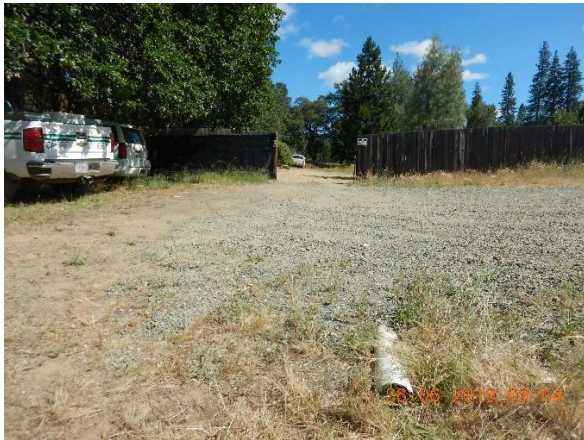
Photo Taken by: Pansy Yuen, 26 June 2019 Photo 51 – North view of the white PVC pipe outlet point, which reappeared under the main access road south of the entrance to the cultivation area. The pipe most likely discharges runoff from the cultivation area.
