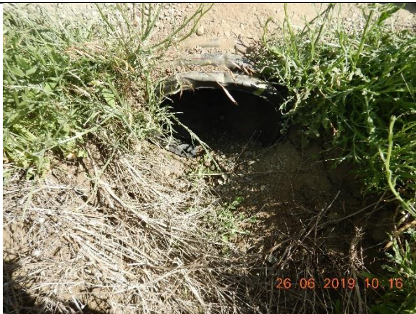
Photo Taken by: Pansy Yuen, 26 June 2019 Photo 59 – North view of a bent culvert with erosion on the access road above the culvert and sediment inside the culvert.
