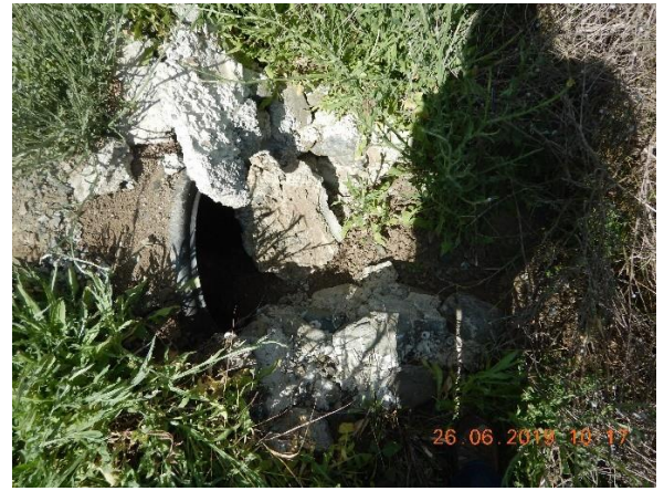
Photo Taken by: Pansy Yuen, 26 June 2019 Photo 58 – Close-up of a culvert outlet point shown in Photo 57 with eroded soil and concrete blocking the outlet.
