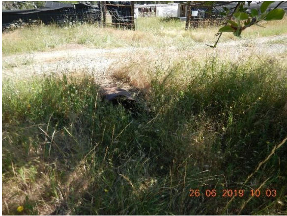
Photo Taken by: Pansy Yuen, 26 June 2019 Photo 55 – North view of a culvert on the south side of the main access road.
