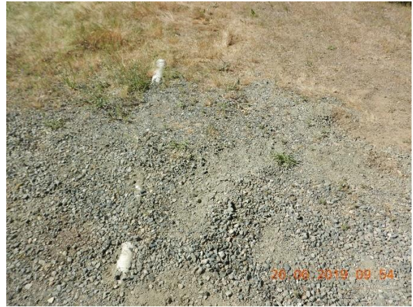
Photo Taken by: Pansy Yuen, 26 June 2019 Photo 50 – North view of a white PVC pipe shown in Photo 49 reappearing south of a main access road.
