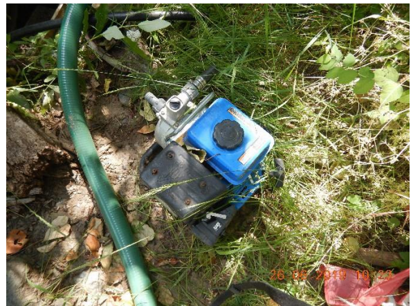
Photo Taken by: Pansy Yuen, 26 June 2019 Photo 64 – Close-up view of a blue water pump next to the galvanized steel corrugated riser pipe.
