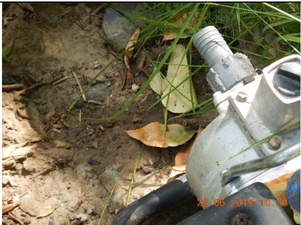
Photo Taken by: Pansy Yuen, 26 June 2019 Photo 65 – Close-up view of a dark stain, most likely an oil stain, under a blue water pump opening. The immediate area around the stain was not wet.
