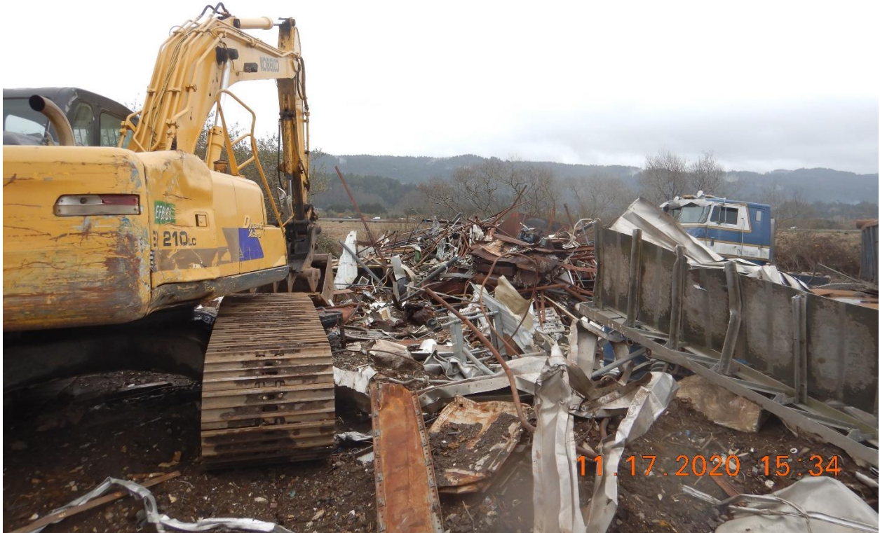
Picture 7 – View of the stored rusty metals by the parked excavator.
