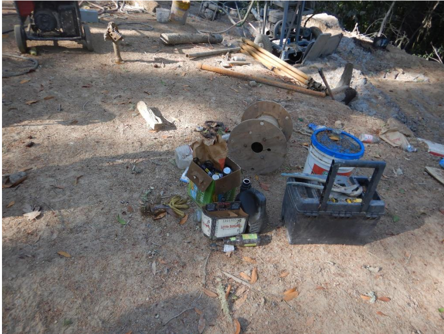
Photo 13—Uncapped gallon jug of hydraulic fluid, among other equipment and materials at WQ 7.
