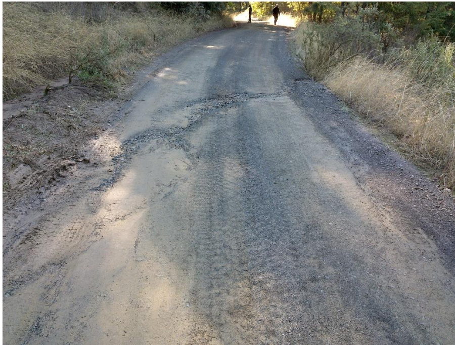
Photo 33—Road in the vicinity of WQ 20. Shows a channel eroded in the road-surface from stormwater originating at WQ 19. Sediment laden stormwater threatens to deliver to a tributary to Sproul creek to the right and out of view of the image.
