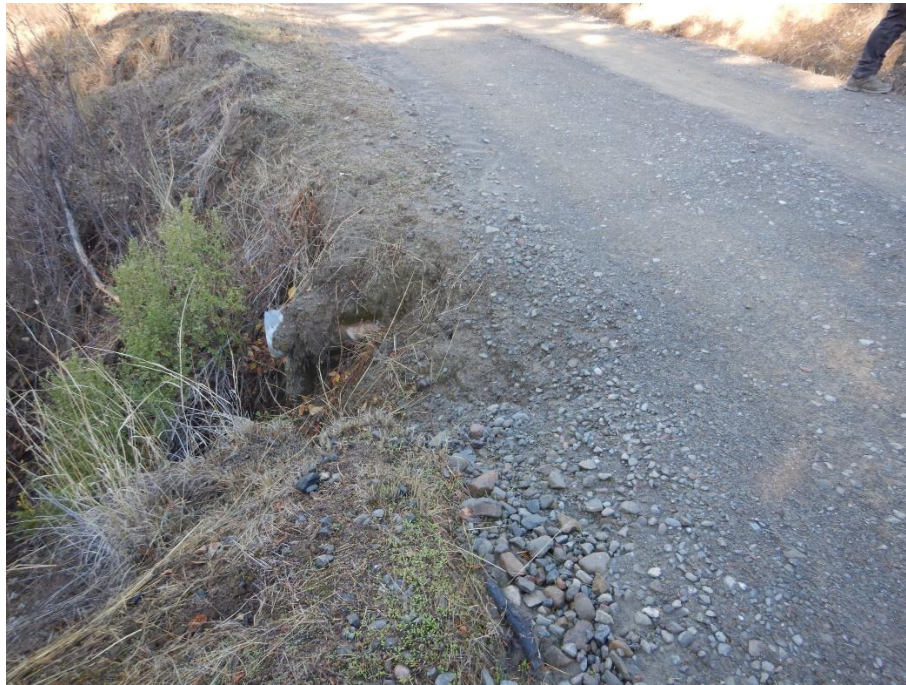
Photo 3—Looking west at culvert outlet located at WQ 3. The culvert is perched, and the channel has incised below the outlet.
