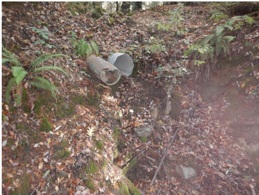
Photo 27—Looking upstream at the two culverts pictured in the previous image perched five feet above the receiving watercourse at WQ 16.
