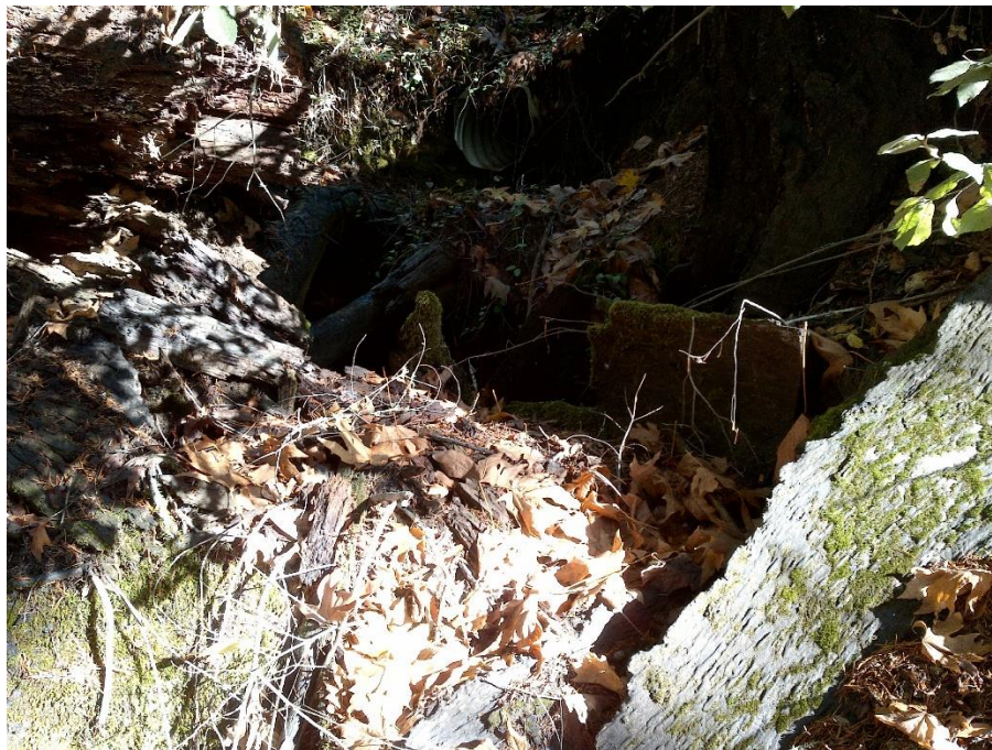
Photo 29—Looking east and upstream at WQ 17 where culvert discharges into the receiving water. The culvert, visible in the top center of the image is perched several feet above the channel.
