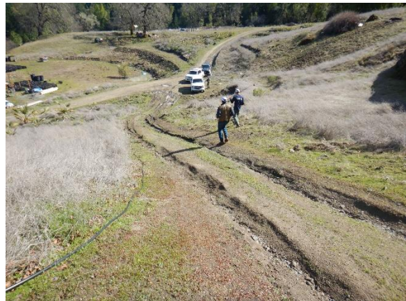
Figure 12. A steep unsurfaced road deliver sediment via rills and stormwater, to the watercourse in Figures 10 & 11.
