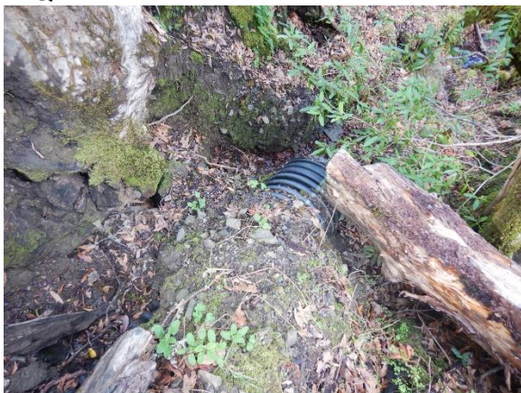
Figure 37. Plugged culvert inlet
