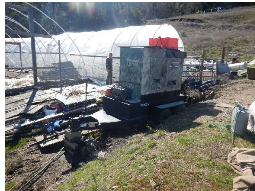
Figure 22. Generator located where runoff could be transported to same watercourse.
