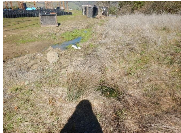
Figure 7. Downstream of the crossings the watercourse is impacted by the construction of a cultivation flat.
