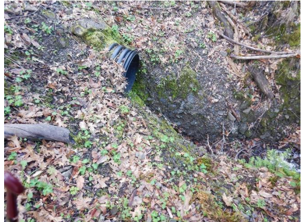
Figure 39. Eroded outlet of culvert.
