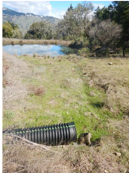
Figure 15. Outlet of Pond 1 to Pond 2.
