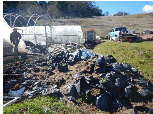
Figure 21. Potting soil and grow bags discarded in a location that waste could be transported to the watercourse shown in previous Figure.
