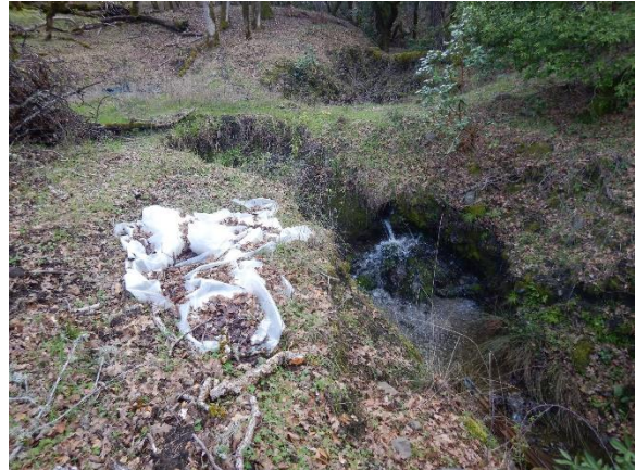
Figure 33. Eroded watercourse crossing, looking upstream.
