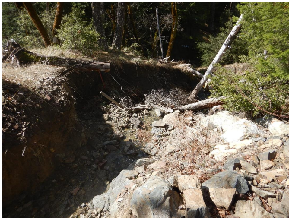
Photo 12—Looking west at northern spillway for Reservoir No. 1. The picture is taken farther downstream from previous image and gully is increasing in depth.
