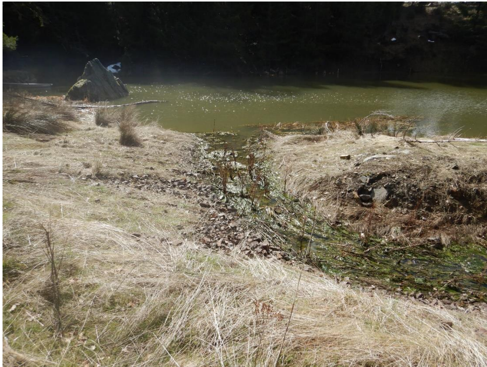
Photo 8—Looking south at northern spillway for Reservoir No. 1 in the vicinity of WQ 3.
