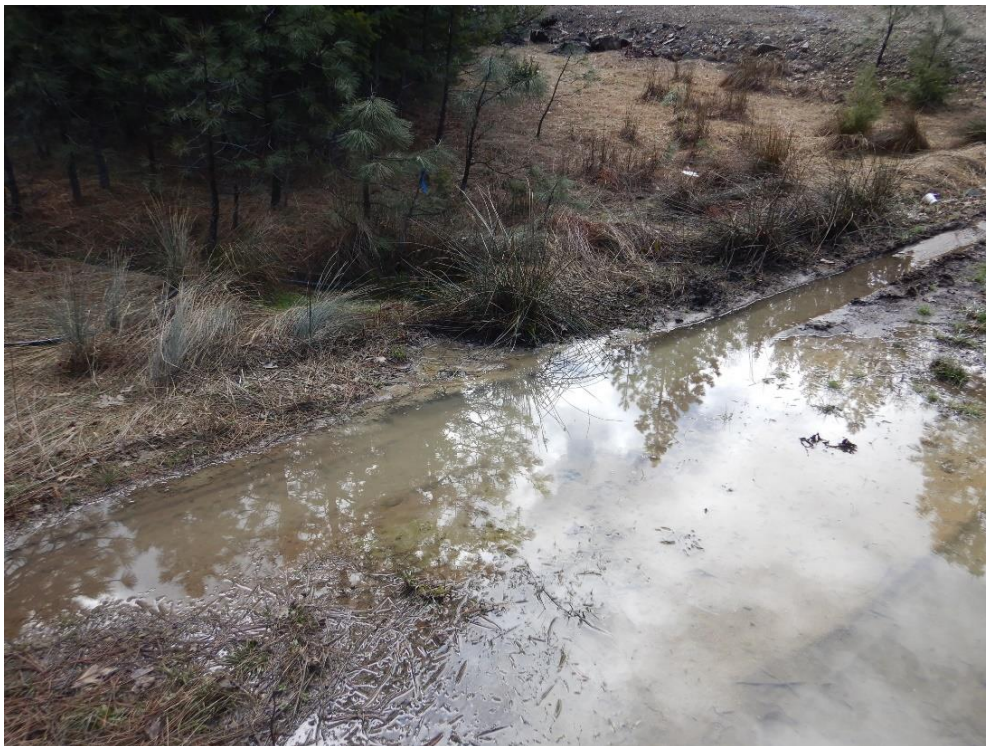
Photo 1—A road flooded at an undersized road crossing at WQ 1.
