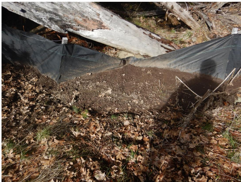
Photo 14—Looking at sediment collected on silt fence at tow of the impounding buttress for Reservoir No. 1.
