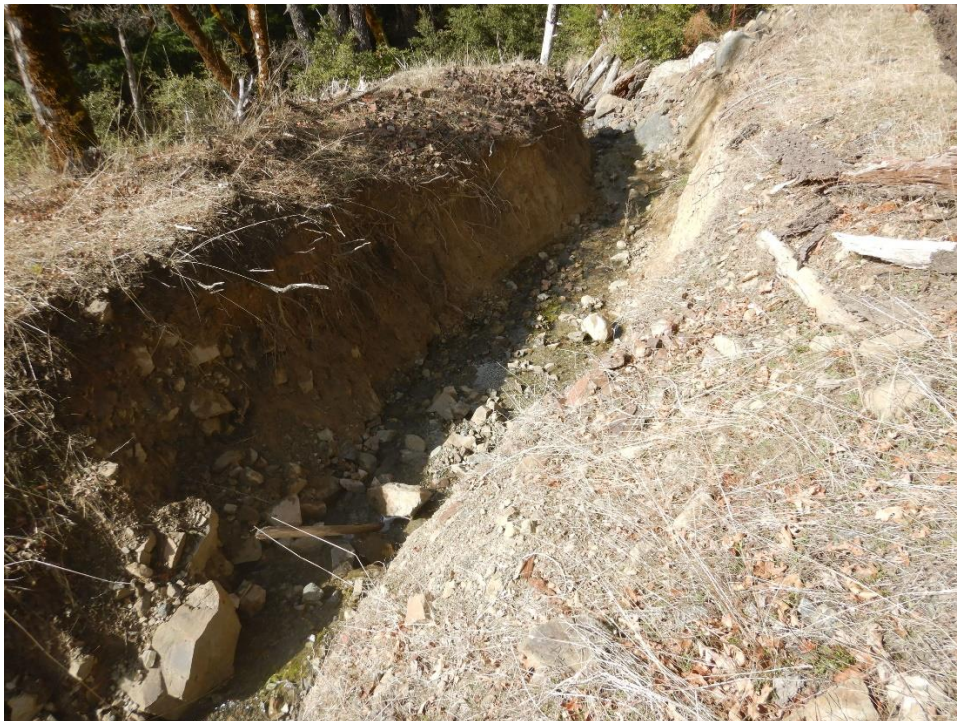
Photo 11—Looking west at northern spillway for Reservoir No. 1. The picture is taken farther downstream from previous image and gully is increasing in depth.
