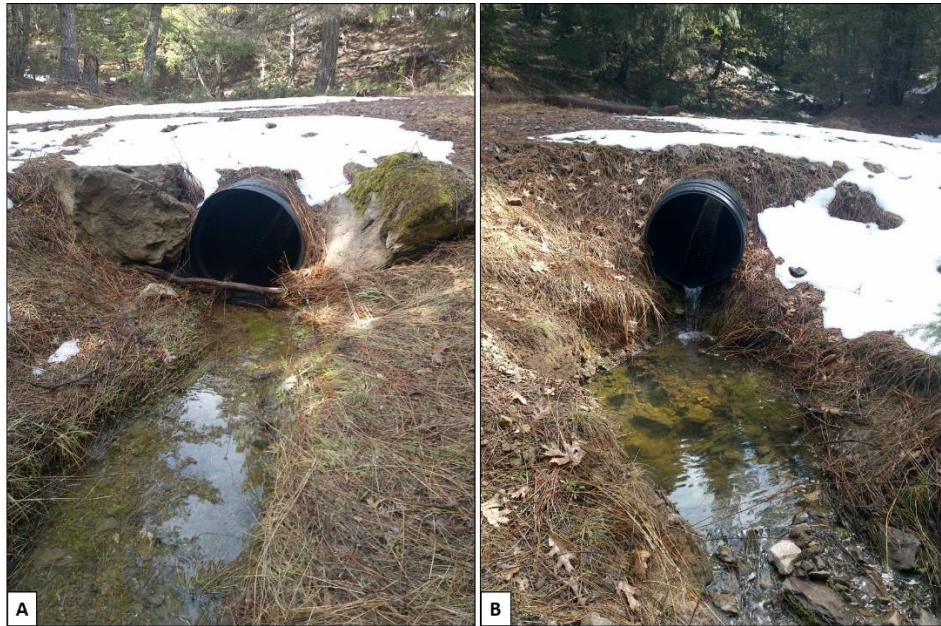
Photo 6—Looking downstream (A) and upstream (B) at culverted watercourse at WQ 2. The culvert is narrower than the watercourse and the outlet is perched 50% of the culvert diameter above the channel bed.
