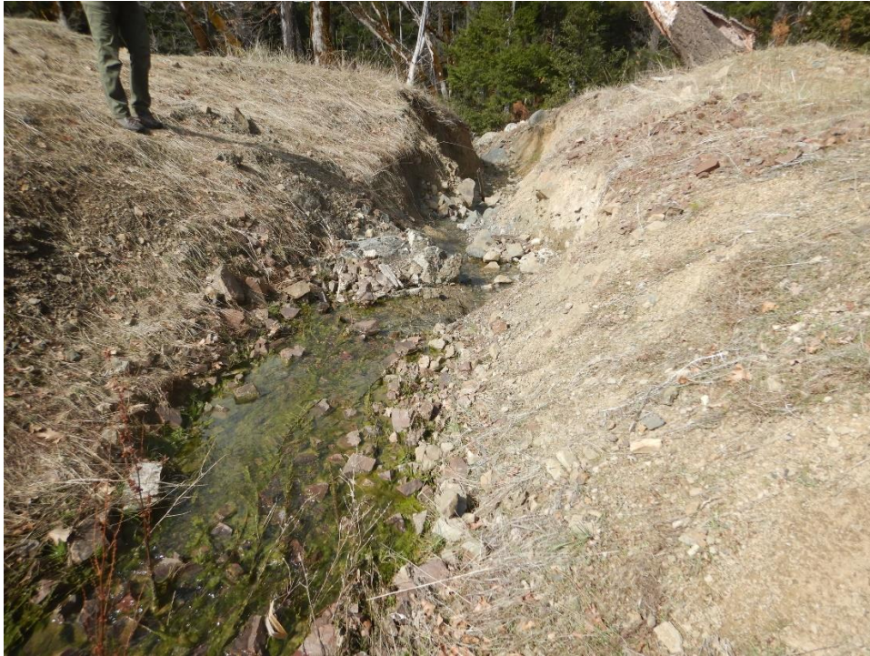
Photo 10— Looking west at northern spillway for Reservoir No. 1. The watercourse is forming a gully near the middle of the image.
