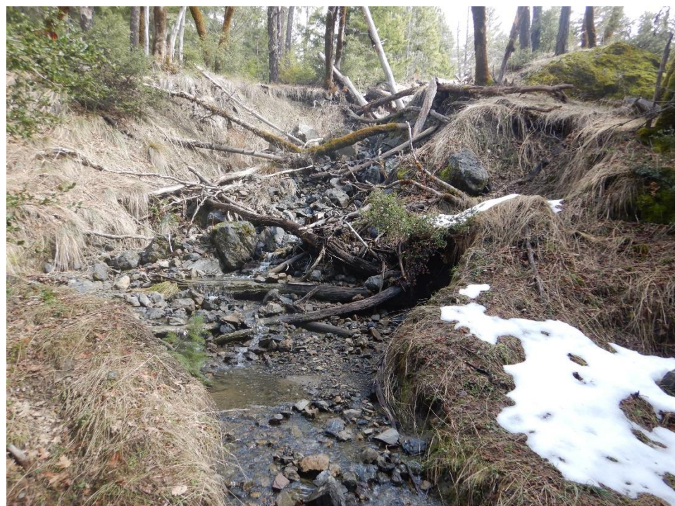
Photo 13—Looking east at northern spillway for Reservoir No. 1. The historical channel downstream from the impounding buttress is to the right of the photographer.
