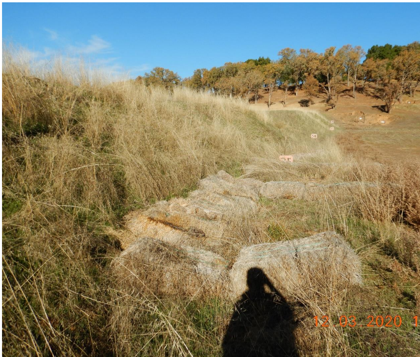
Picture 8- View of a vegetated swale along the west side of the main range area. Several hay bales are installed along the swale. The runoff is discharged into a protected inlet at the low point and drains through a pipe via a culvert. Located in DA-2. Picture taken by Farzad Kasmaei.
