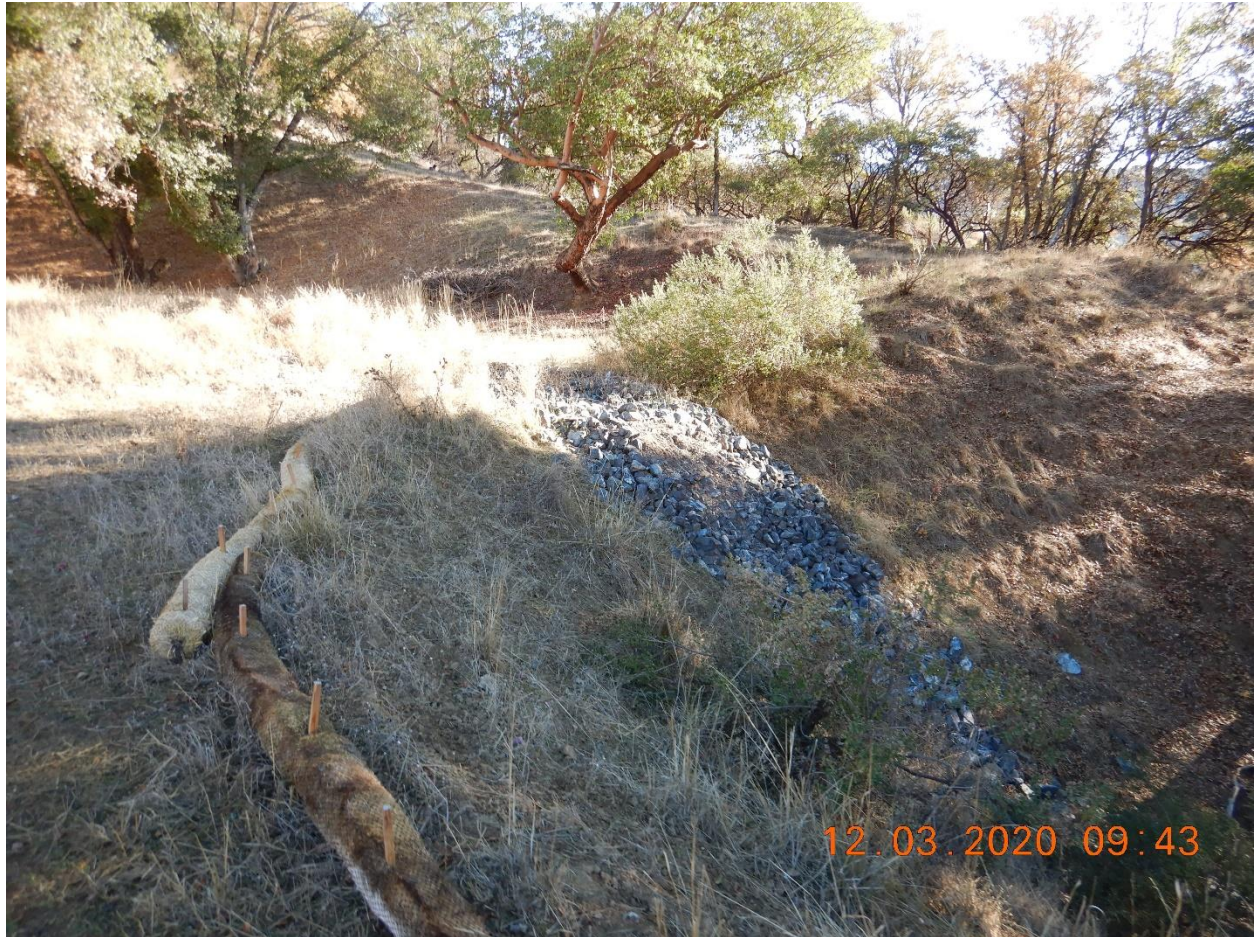
Picture 3- View of the riprap area within Drainage Area 1 (DA-1) where the runoff is discharged on the hill side.
