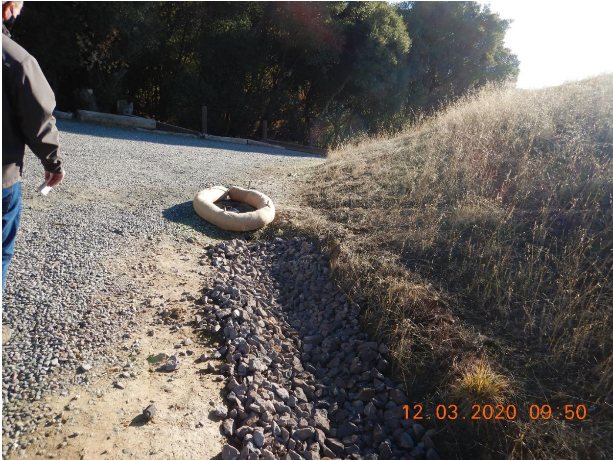
Picture 5- View of the rock lined drainage ditch and the protected inlet in DA-1.
