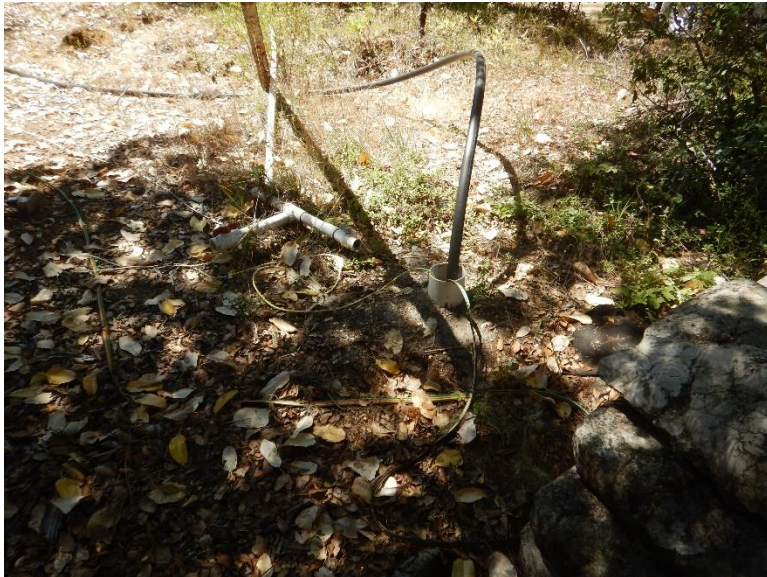
Photo 2: Well: Unsealed groundwater well
