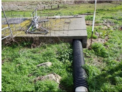
Flexible pipe conveys milk barn wash water and some corral runoff to waste tank.
