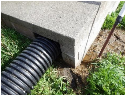
Flexible pipe outlet in west side of waste tank inlet. Note runoff on right.
