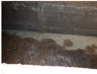
Liquid level inside waste tank showed about 18 inches of freeboard before reaching level of flexible pipe inlet opening
