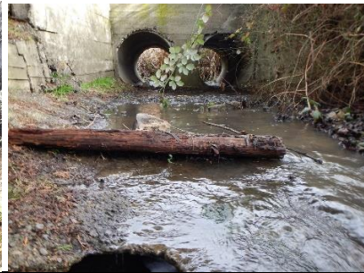
Estero de San Antonio Creek outlets of two 4' diameter driveway culverts
