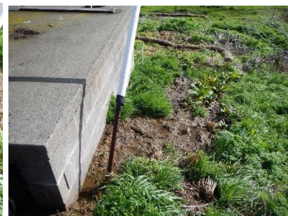
View of south side of waste tank. Note waste runoff accumulation.
