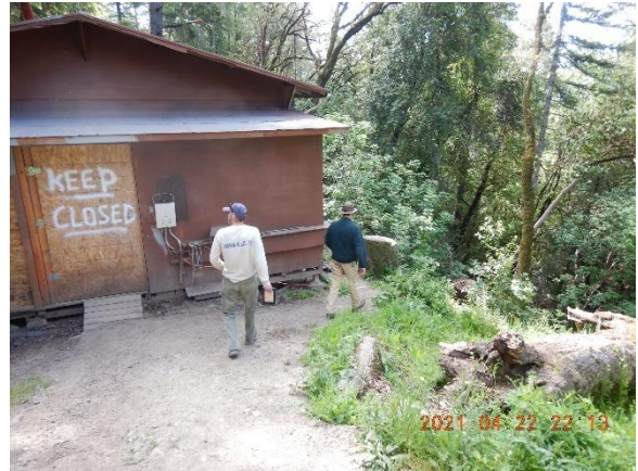
Figure 13. Building built at edge of slope, with south west corner may be in riparian setback of large class II watercourse.
