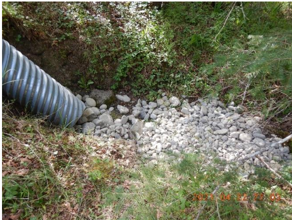
Figure 8. Rock recently placed in void in scoured channel. Rock is too small to stay in place.
