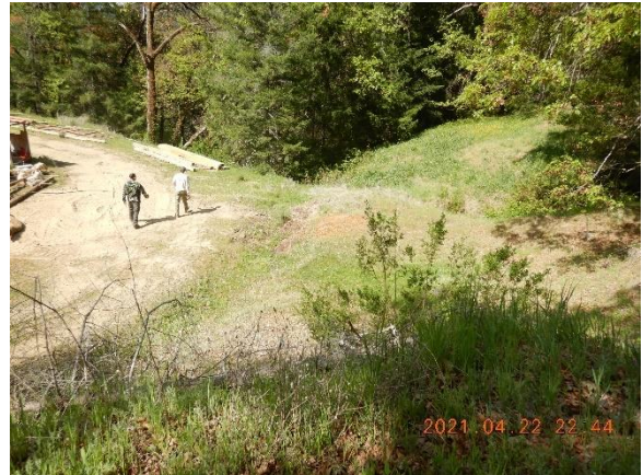
Figure 22. Landing built in riparian setback, to be pulled back and Class II riparian setback to be restored.
