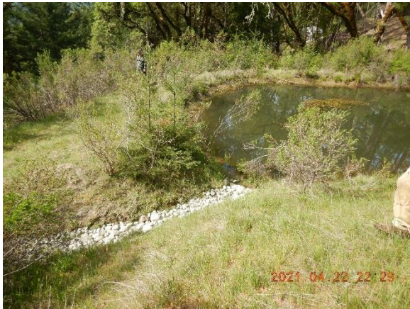
Figure 20. WQ6, pond outlet with recently placed rock which is too small to stay in place.
