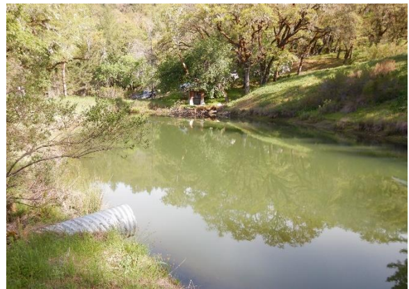
Figure 5. Pond at overflow pipe, minimal free-board.
