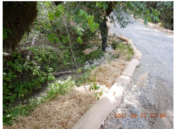
Figure 10. The scoured channel runs parallel to the road and then goes into an undersized culvert; the alignment could be improved away from road. Recent erosion control measures including rock placed in channel at inlet. Rock is too small to stay in place.
