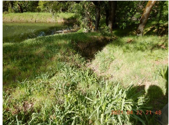
Figure 4. Scoured channel downstream of road and upstream of pond.
