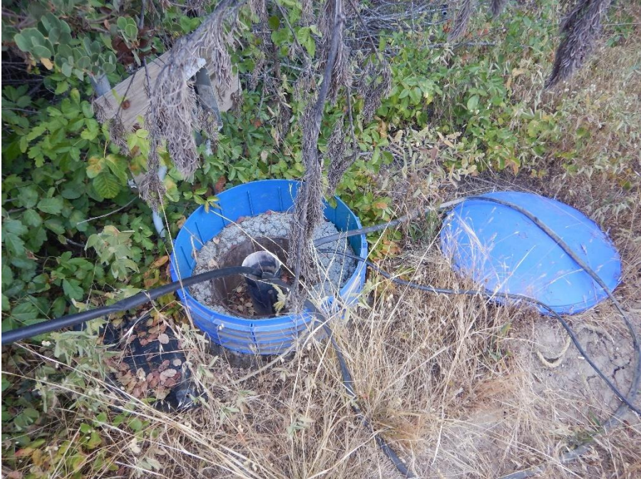
Photo 3: Unsealed groundwater well
