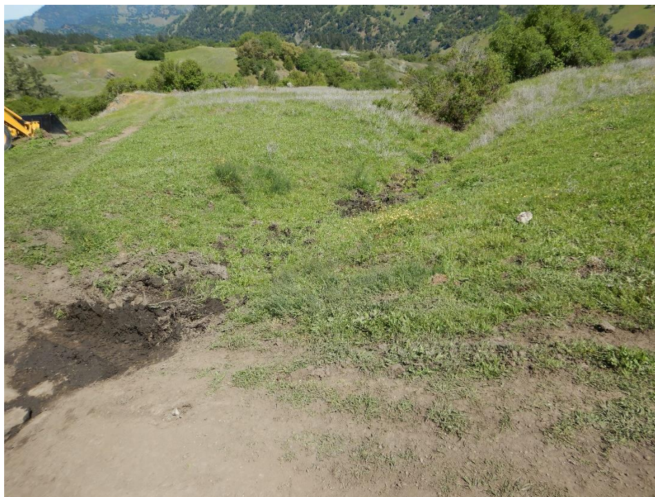
Photo 29—Looking north where saturated ground pictured in previous image connects to a watercourse tributary to the Eel River.
