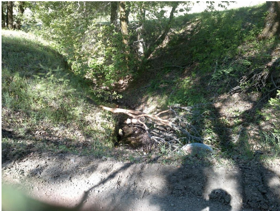
Photo 8—Looking upstream at a 36-inch diameter corrugated metal pipe upstream from the tank in the previous image, in the vicinity of WQ3. The culvert inlet is misaligned with the watercourse.
