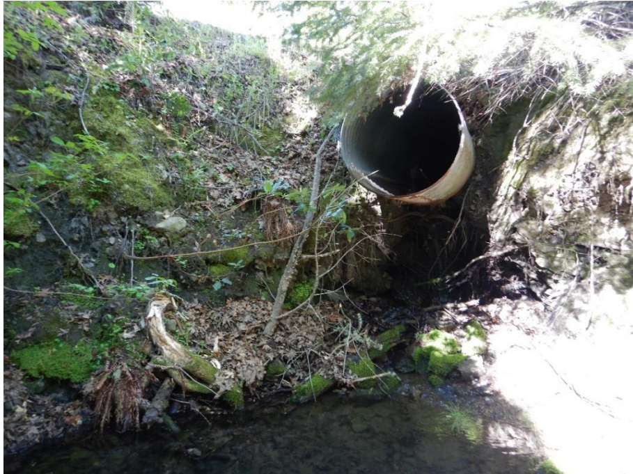
Photo 9— Looking upstream at outlet of culvert pictured in previous image at WQ3. The culvert outlet is perched 5 feet above the stream bed and has rusted through the bottom.
