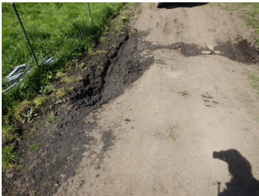
Photo 28— Saturated ground on the road passing the northern edge of the graded pad at WQ7.
