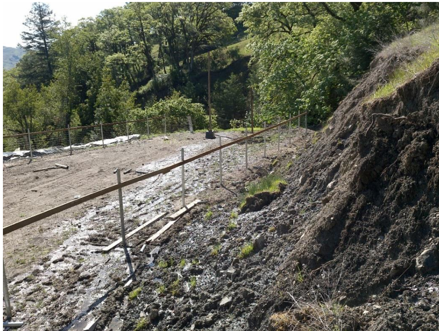
Photo 14— Looking southeast along graded pad south of WQ4. The photographer is standing at the same location as the previous two images. Water emanates from cut-face and flows over cultivation pad to receiving water in the background of the image.
