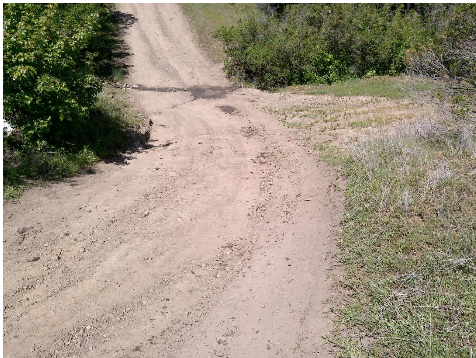
Photo 40—Hydrologically connected road fording a watercourse north of WQ10.
