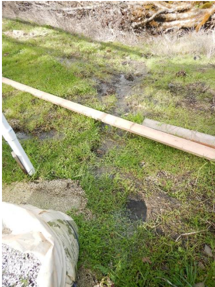
Figure 12. View to riparian setback with perlite accumulation from stormwater transport with flow path from greenhouse to fillslope and watercourse.
