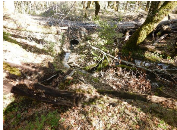
Figure 6. Crossing near tanks (399). Road is eroding and contributing sediment to watercourse.
