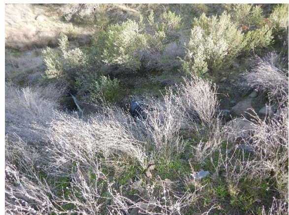
Figure 16. Pond B outlet pipe delivers to a watercourse.
