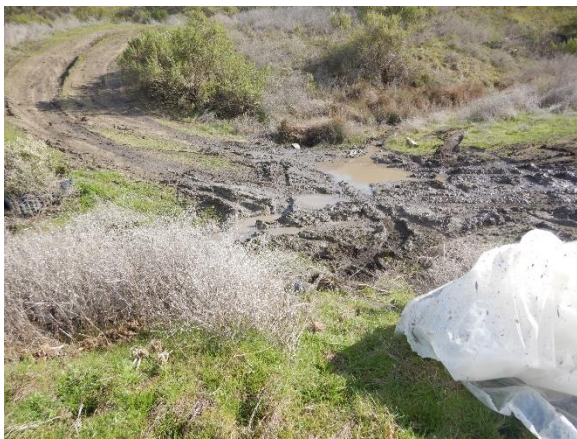
Figure 13. Undersized stream crossing accessing cultivation flat contributes sediment to watercourse.
