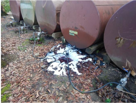
Figure 3. Fuel leak at fuel storage area next to building.
