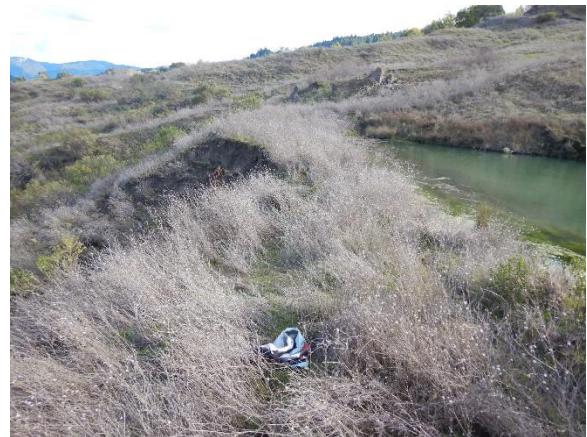
Figure 15. Erosion void on Pond B.
