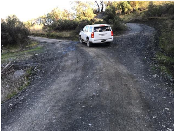
Figure 23. Convergent roads at watercourse crossing are hydrologically connected to watercourse and deliver sediment to watercourse.
