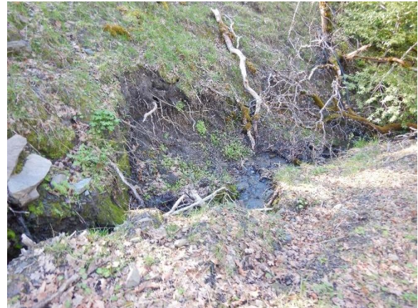
Figure 10. Downstream of outlet discharge, channel is eroding along toe of berm.
