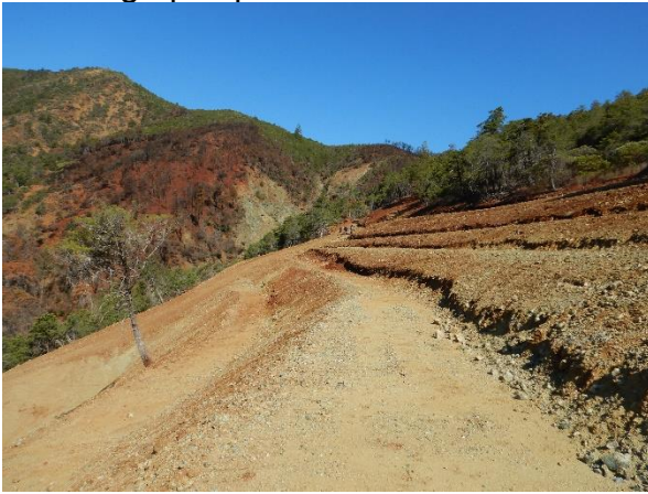
Photo 3: View of unstable hillside terracing upslope from WQ2.
