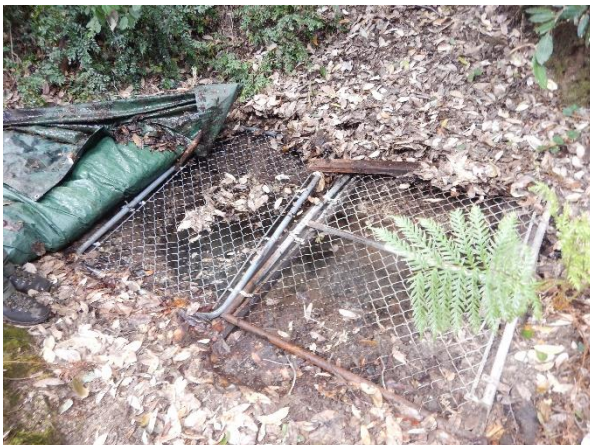
Photo 11: Point of diversion infrastructure at SPRG2.
