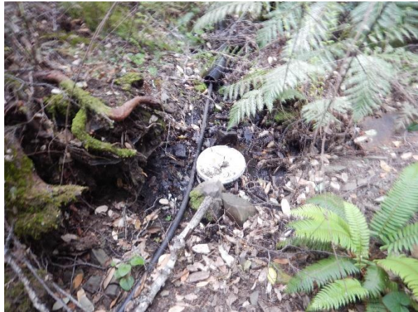
Photo 10: Point of diversion infrastructure at SPRG1.
