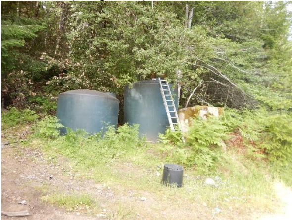
Photo 9: Water storage tanks located near the spring complex
