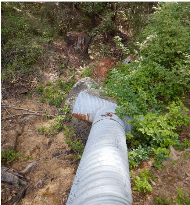
Photo 3 - Cultivation Area 1: Culvert discharges to head of Class III watercourse. Fine sediment is visible around the culvert outlet
