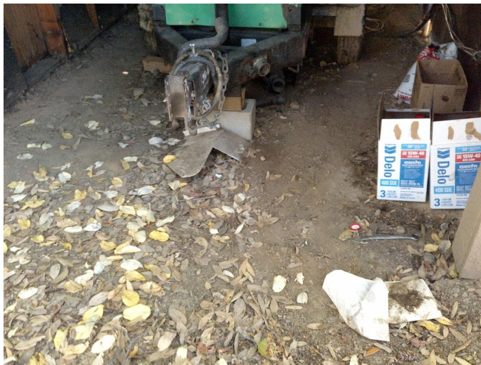
Photo 3—Generator building located at WQ3. The generator lacks secondary containment and the building has an earthen floor.
