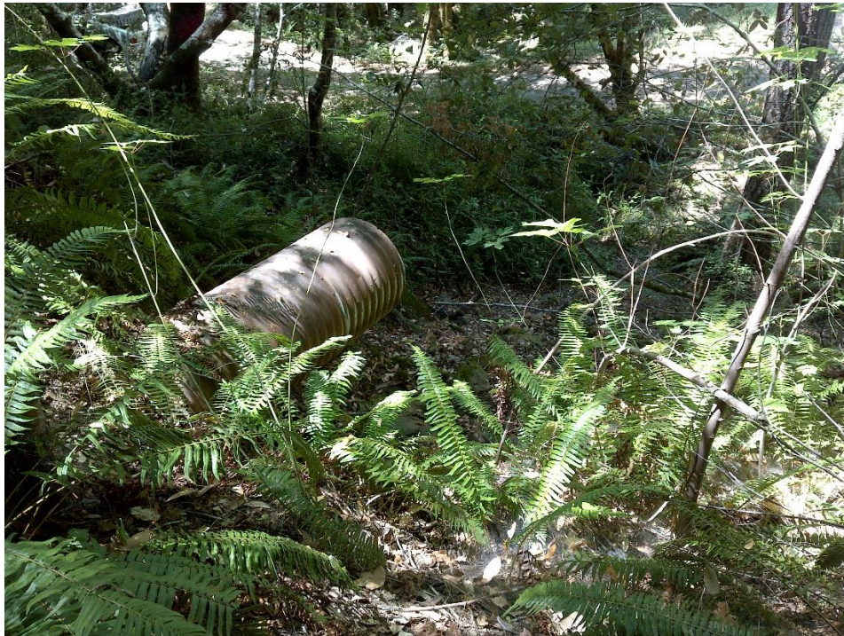
Photo 8—Culverted road crossing located at WQ4. The culvert is two feet in diameter and the outlet is perched four feet above the channel below.
