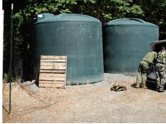
Photo 8: water storage tanks at WQ8
