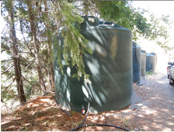
Photo 3: water storage tanks at WQ3
