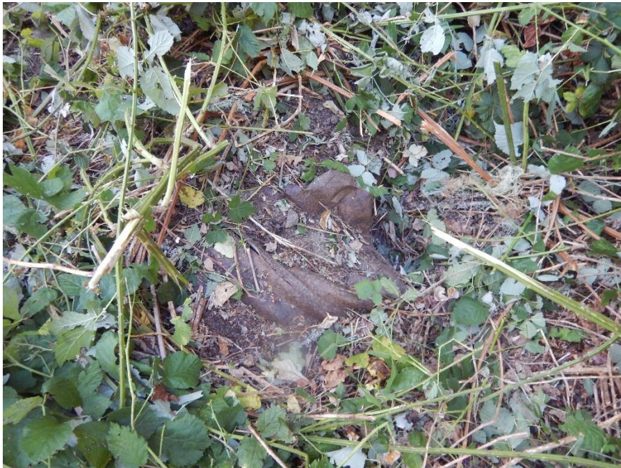
Photo 4: GG4: Squashed, rusted culvert inlet
