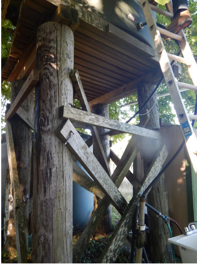
Photo 1: GG1: Two water tanks with leaking connection
