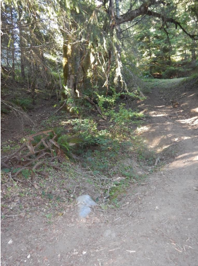
Photo 7: GG7: Misaligned culvert receiving flow from a Class III watercourse and road runoff
