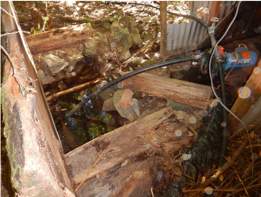
Photo 10: GG10: Shed, pump, and black poly diversion line in spring above pond
