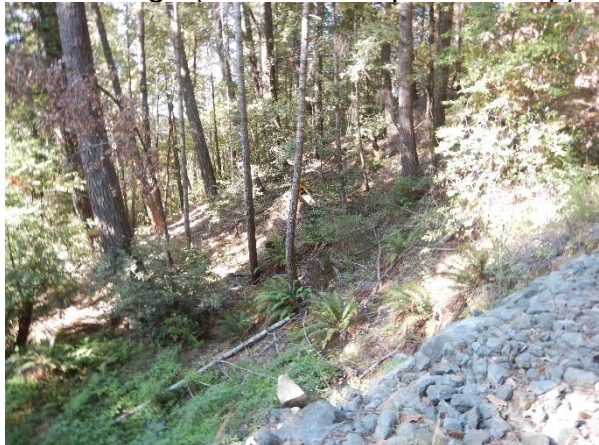
Photo 16: Downslope view of the head of the drainage (ROAD on Inspection Map)
