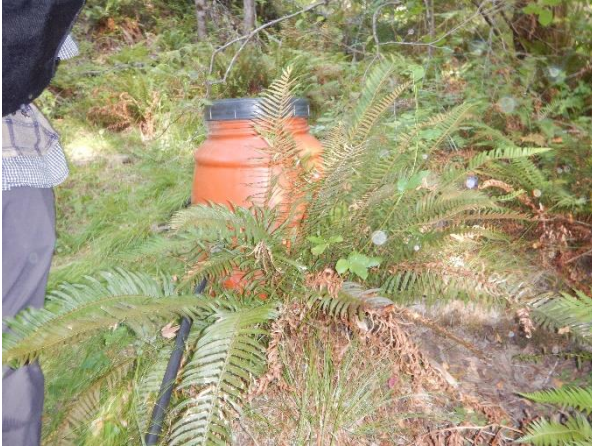
Photo 19: Assumed settling tank located down slope of the POD.
