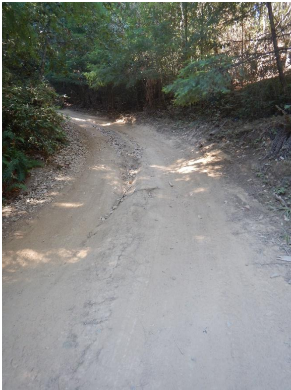
Photo 4: Access road with surface erosion
