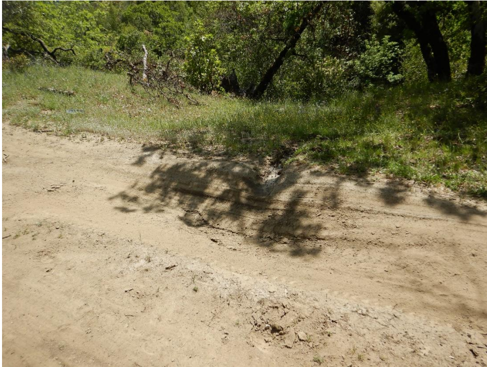
Photo 3—Looking north at scour marks on the edge of road west of WQ1. The watercourse leading to WQ1 is out of view in the background of the image.
