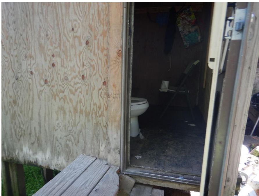
Photo 26—Toilet discharging to ground adjacent to watercourse east of WQ6.
