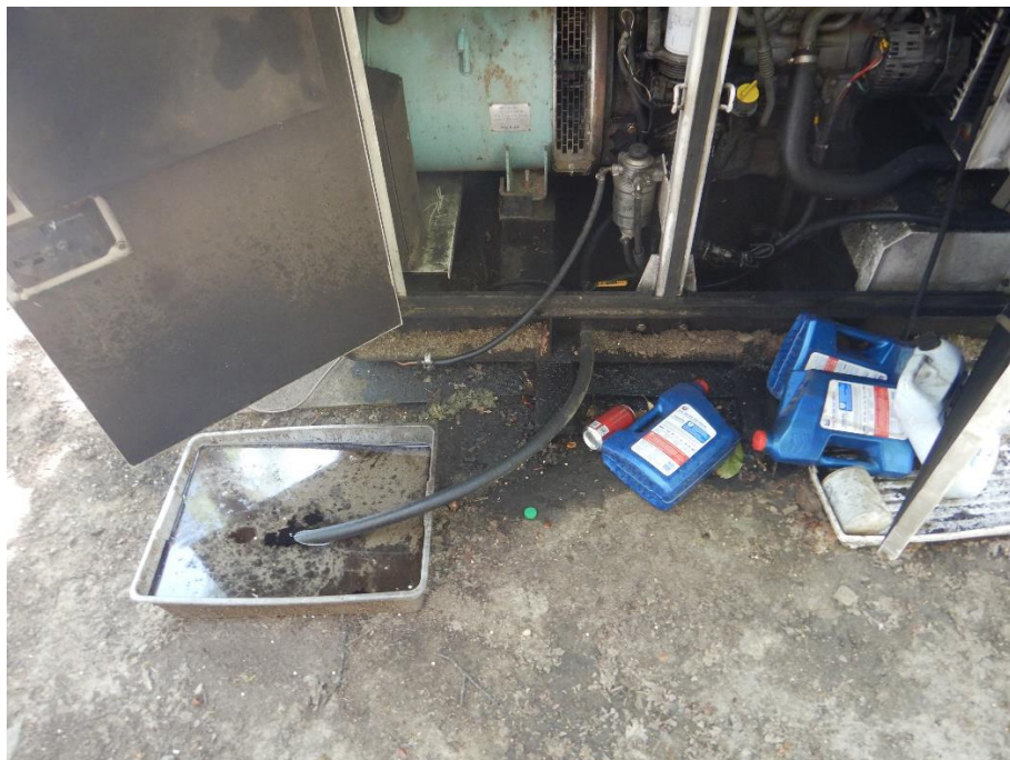
Photo 20—Motor oil leaking out of diesel generator at WQ4. Patch of dark earth below the generator identifies the location of an oil spill.
