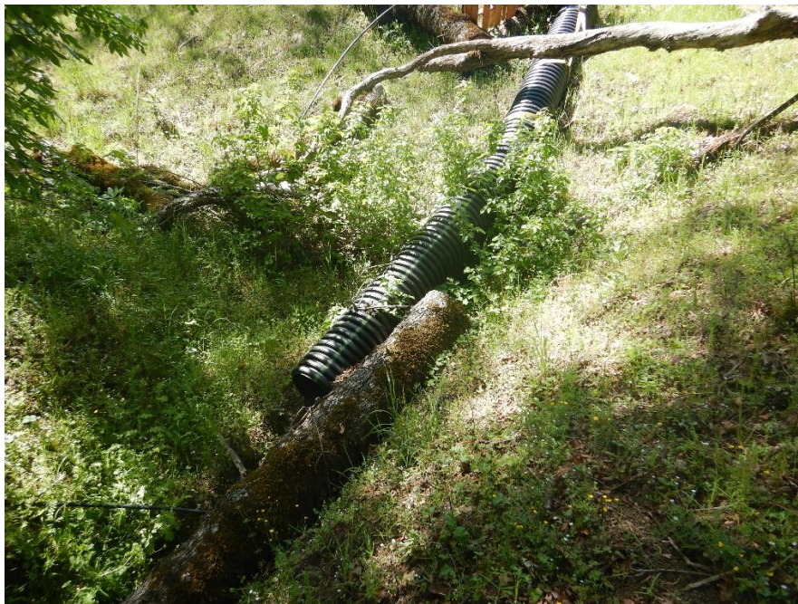
Photo 24—Looking west at the reservoir outlet pipe. The pipe is resting on a cut and fallen tree.
