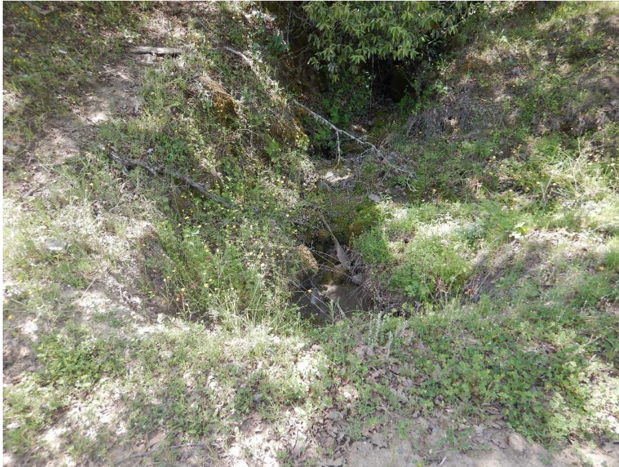
Photo 1—Looking west at watercourse upstream from culvert crossing at WQ1. Staff estimated that the active channel is four-feet wide. A roadside ditch discharges to the culvert inlet from the road to the north as well.
