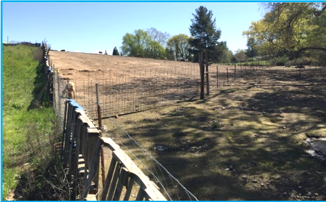
Photograph 8. March 25, 2021. Standing at the bottom of the hill and adjacent to the Woody Creek fence and looking up the hill. The barren buffer strip can be seen to the right of the photograph between the new setback fence and Woody Creek top-of-bank fence. The draft LandSmart Plan recommends the buffer strip be covercropped. Additionally, the Southwest Pasture was 100% exposed soil and absent any vegetation.
