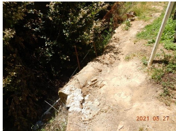
Figure 11. Fill pushed over logs at CA2 in attempt to increase surface area of cultivation area.
