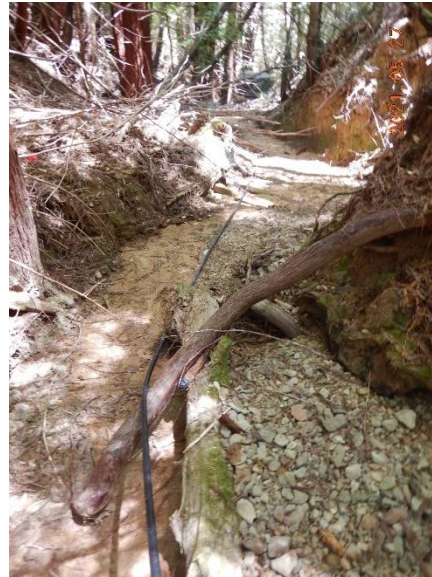
Figure 21. WQ2. Upstream extent of sediment deposition in watercourse. Note clean gravels on right and on left and down channel is buried in discharged fine sediment.
