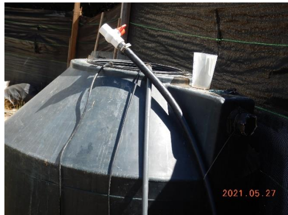
Figure 5. Feed tank and waterline in at CA1.
