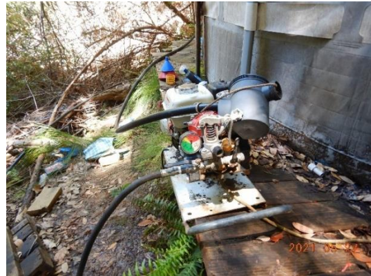
Figure 26. Gas pump without containment.
