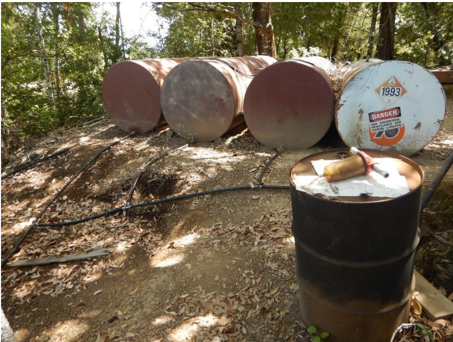
Photo 6: LL4: Four fuel tanks connected to pump handle
