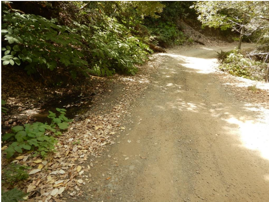
Photo 10: LL8: Ponded water in inboard ditch from hillside seep
