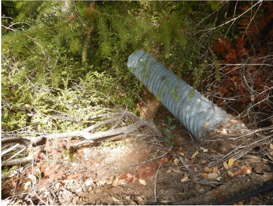
Photo 9: LL7: Culvert stream crossing with perched outlet
