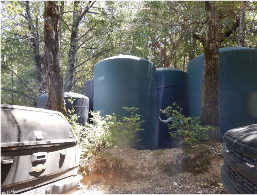
Photo 1: LL1: Water storage tanks
