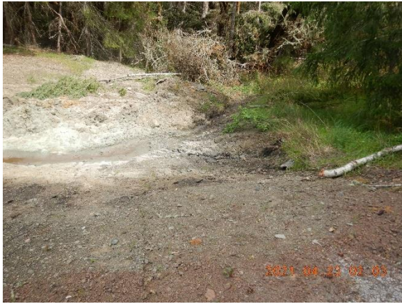
Figure 4. Downstream of watercourse filled with sediment and slash at GPS location 489.
