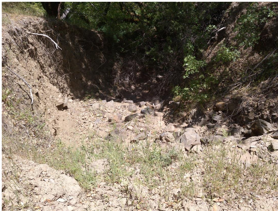
Photo 19 Looking downstream where a road fords a four-foot wide dry watercourse at WQ10.
