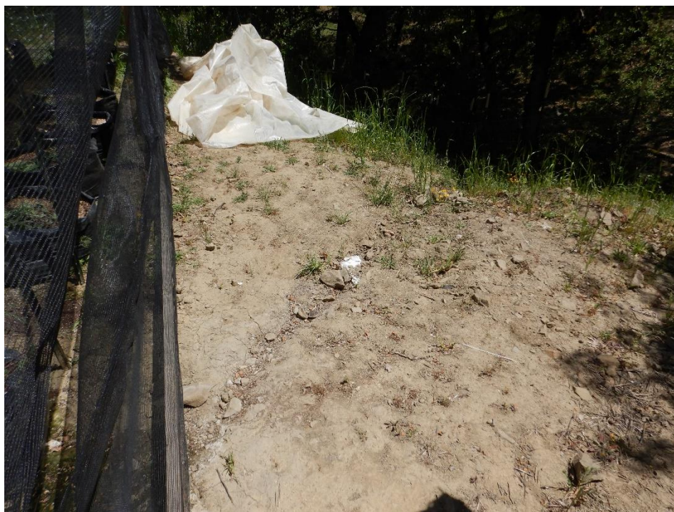
Photo 24—Southern edge of greenhouse pictured in previous image. A trench can be seen leading towards a watercourse obscured by shadows in the background of the image.
