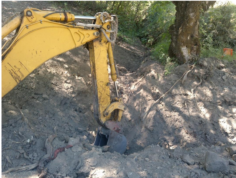
Photo 15—Backhoe at excavation site on road at WQ8. A watercourse can be seen approaching the work area in the background of the image.
