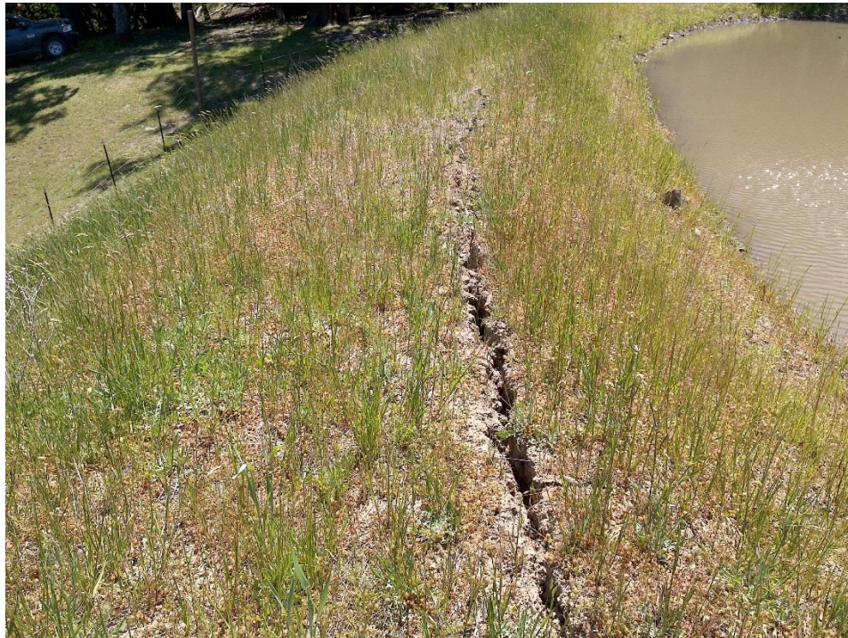
Photo 28—Tension crack along the reservoir's berm at WQ13.
