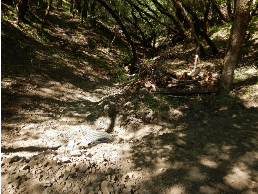
Photo 1—Looking east and upstream at recently installed watercourse crossing at WQ1. The inlet for the 24-inch diameter culvert is visible in the lower left of the image. The watercourse upstream has an approximate four-foot-wide active channel width.
