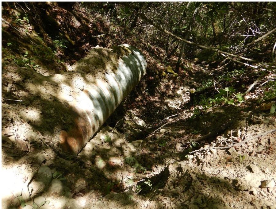
Photo12—A 24-inch diameter culvert at WQ6. The culvert outlet is perched approximately three feet above the receiving watercourse's bed. Staff estimated that the active channel upstream from the culvert is three feet wide. Two new 24-inch diameter pipes were staged nearby for suspected replacement.
