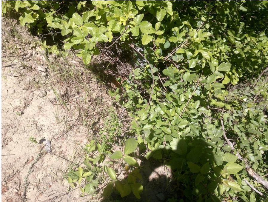
Photo 13— An approximate 24-inch diameter culvert at WQ7 is perched above the receiving watercourse's bed. Staff estimated that the active channel upstream from the culvert is between three and four feet wide.
