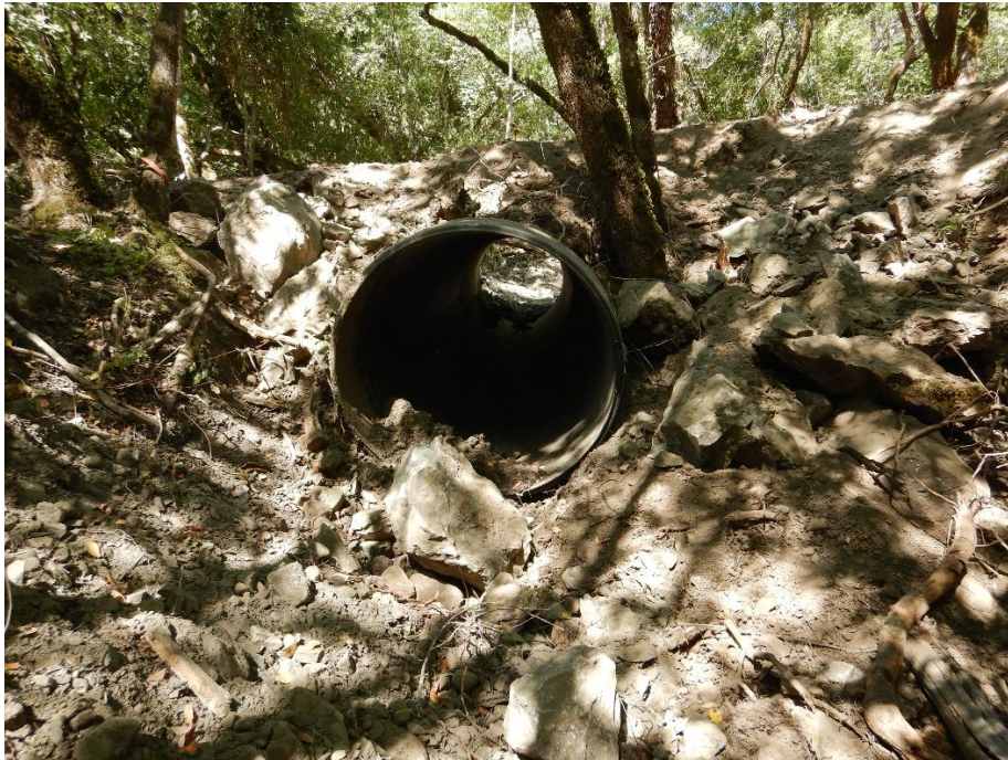
Photo 6—Looking downstream at inlet to newly installed 60-inch diameter culvert installed in the vicinity of WQ2, upstream from the channel pictured in Photo 4 and Photo 5 above.
