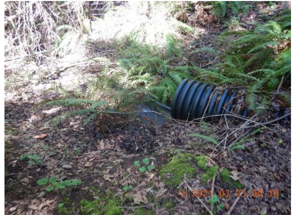
Figure 5. GPS point 445, inlet of 24" which is misaligned located on a Class II watercourse, on a road behind residence, road does not appear to be in use. The culvert was not disclosed in LSA.
