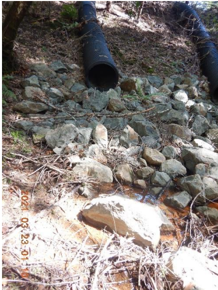
Figure 19. The separated pipe was not flowing water but I observed water between the rip rap at the outlet, indicating seepage at pipe separation or berm seepage.
