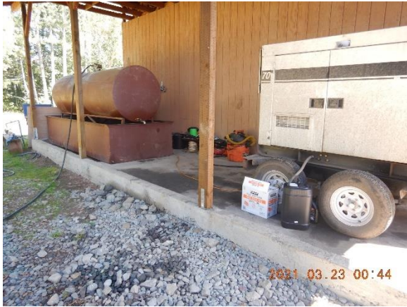
Figure 11. GPS location 447. A large generator powers the three large greenhouses. Indications of numerous small spills, as assessed by HumCo HazMat.
