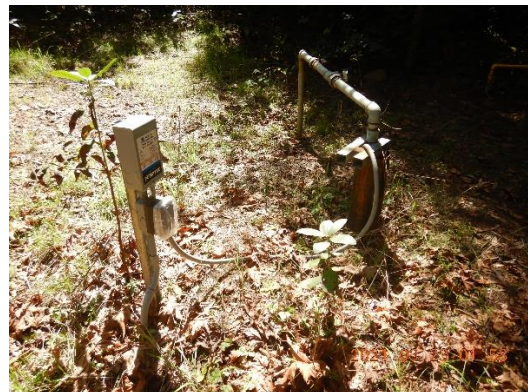
Figure 26. GPS location 461. Well without proper cap.
