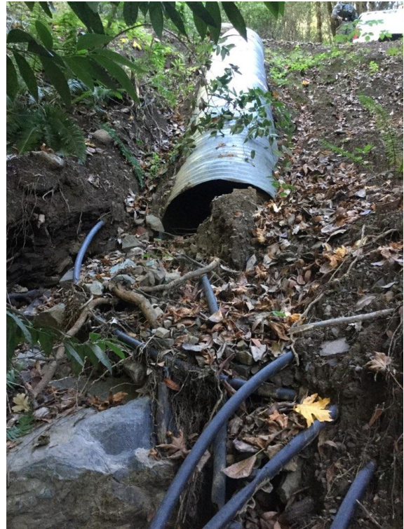
Figure 25. Photo of Crossing 1, by Ryan Bourque of CDFW taken on December 7, 2020 inspection. Photo shows lack of erosion control and erosion and sediment transport to the watercourse at the outlet of the downspout.
