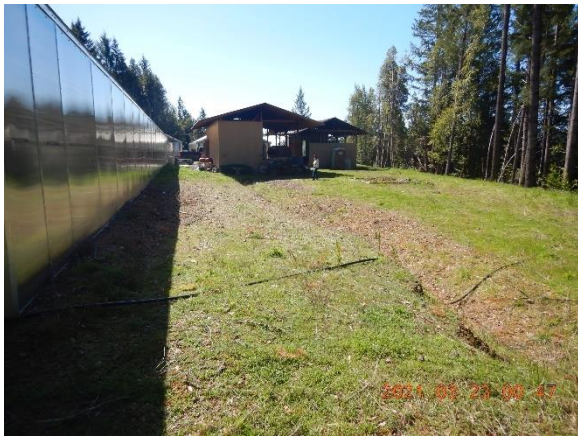
Figure 12. GPS location 448. Gutters catch approx. 12,000 sq ft of greenhouse roof runoff and route it to a trench, located on back side of fuel storage and generator area shown in previous figure. Runoff from the generator area could transport to the trench.
