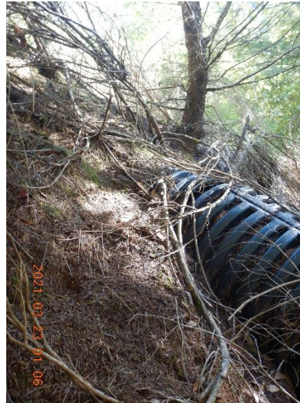
Figure 17. GPS point 454. One of the pond outlet pipes is separated at the 45, near the top of the berm
