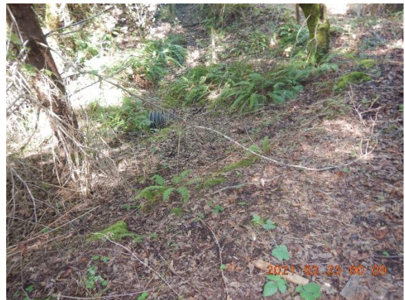
Figure 6. Outlet of culvert at GPS Point 445.
