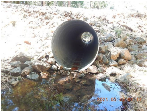
Figure 20. GPS location 455, LSA Crossing 3. Downstream of pond, the stream crossing Culvert was upgraded in ~2018, while enrolled in cannabis general order, without first obtaining authorization for instream work from the Regional Water Board. The inlet is a bit
