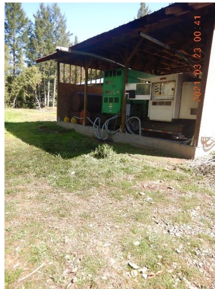
Figure 10. Generator at GPS location 447.
