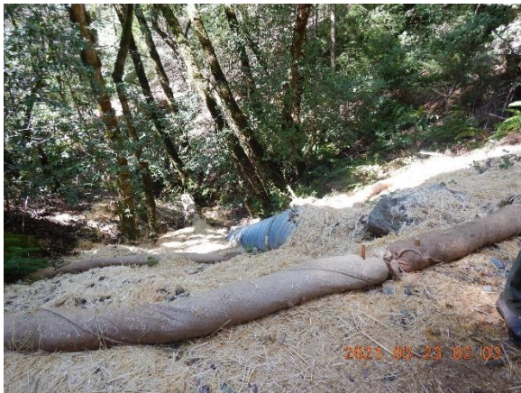
Figure 24. GPS location 462. Crossing 1. Downspout was included in the LSAA but was added during installation of the 36" culvert.
