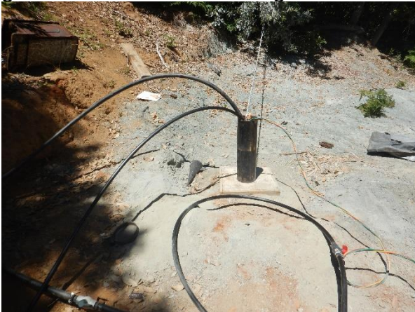
Photo 17: View of the open, uncovered groundwater well and drilling materials.
