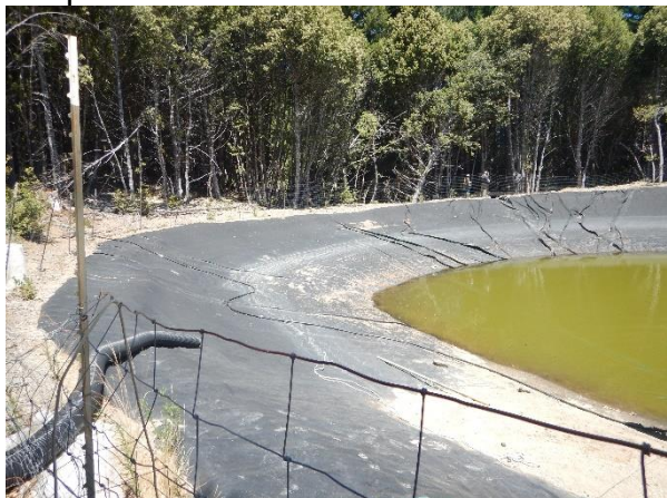
Photo 6: View of the pipe discharging into the pond and sediment delivered.
