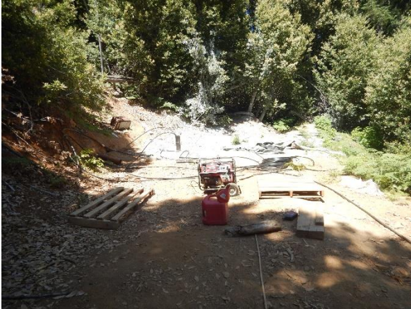
Photo 15: View of the groundwater well and associated generator.
