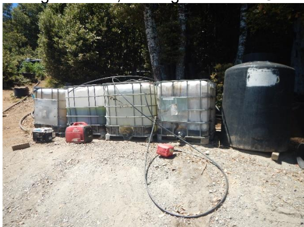
Photo 12: Multiple tanks for storing and mixing nutrients, and a generator at CA1.
