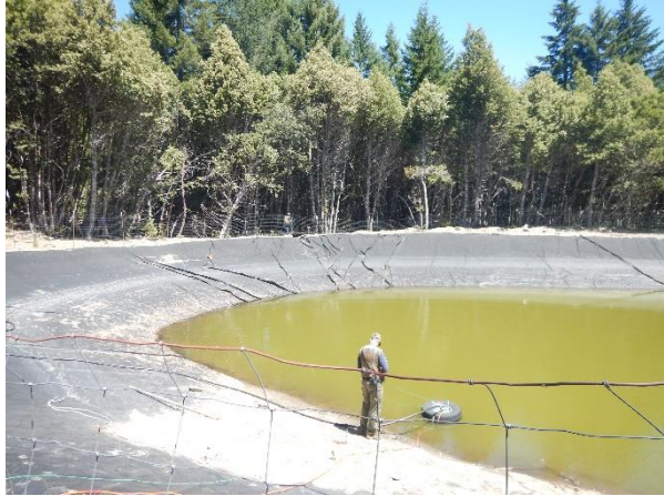
Photo 8: View of the sediment from pipe discharging to the pond and pump.
