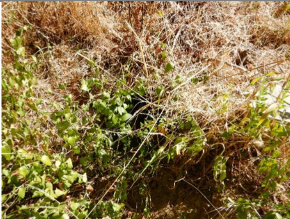
Photo 7: partially clogged pond overflow at inspection point WQ5.
