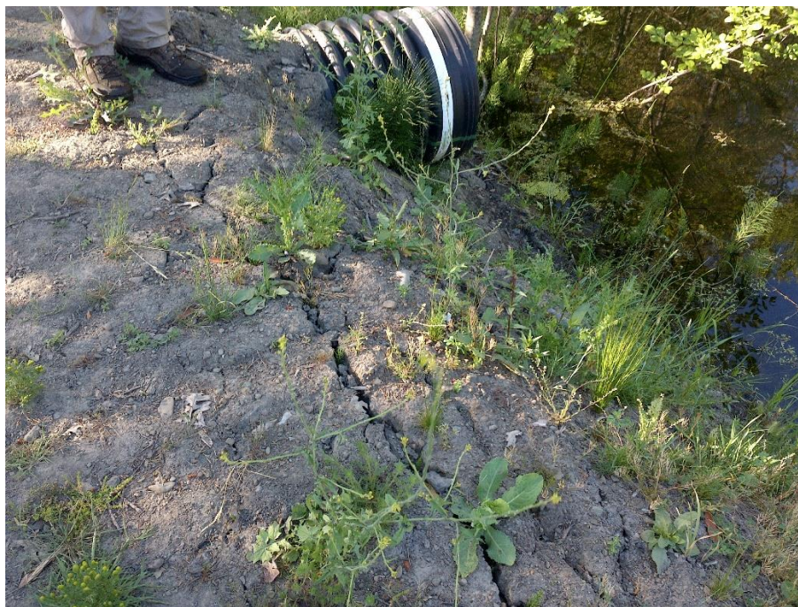
Photo 3— Tension cracks visible on the reservoir buttress at WQ1.
