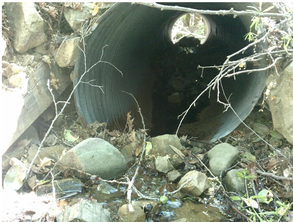
Photo 28—Looking downstream at the inlet of a 32-inch culvert at WQ 9. Staff observed the watercourse upstream was significantly wider than the culvert. A small boulder is visible inside the culvert near the outlet.
