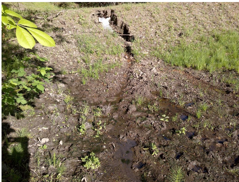
Photo 16—Looking north at outboard face of southwestern reservoir buttress. Water is flowing from a cavity in the earthen buttress.
