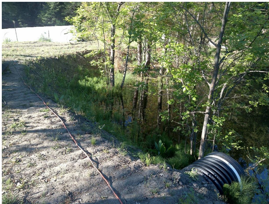
Photo 1—Looking south along reservoir buttress from WQ1. Equipment tracks are evident on the buttress surface and living trees are inundated inside of the expanded reservoir.
