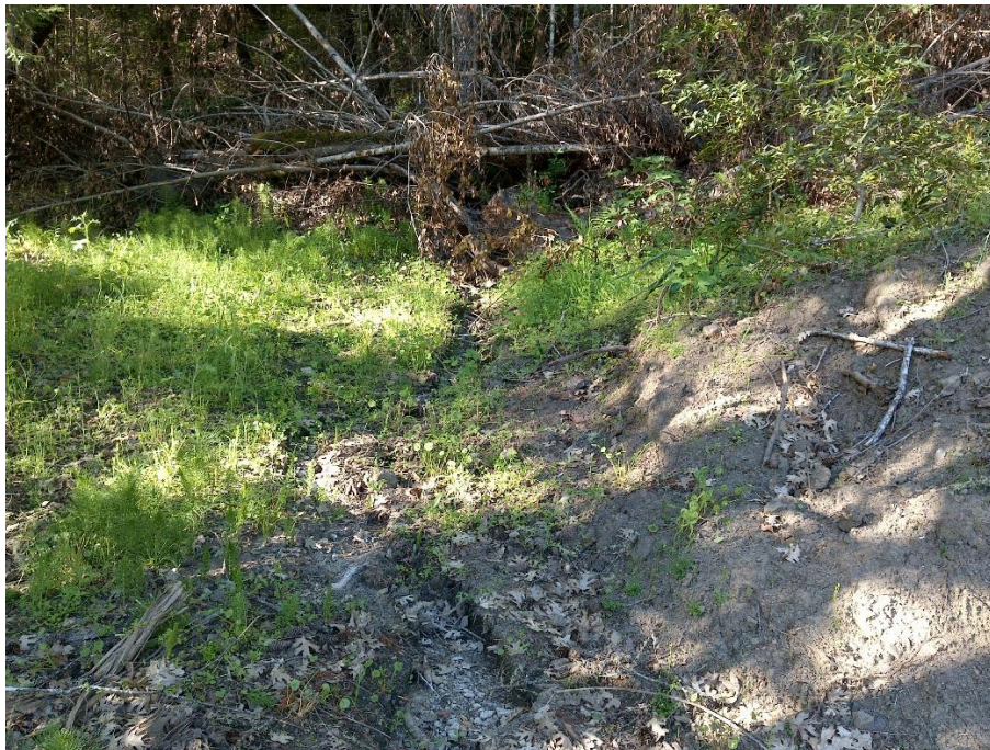
Photo 14— Closer view of southwestern berm visible in the center of the previous image. An incised channel is visible in the center of the image indicating surface water from the upstream drainage had concentrated and scoured the earthen surface of the recently constructed berm.
