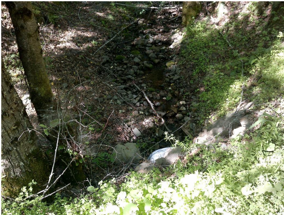
Photo 30— Looking downstream from WQ 9. The culvert outlet is visible in the foreground of the image. The watercourse has a steep right bank, duff covered flood plain along the left bank and a small boulder and large cobble substrate in the wetted portion of the channel.
