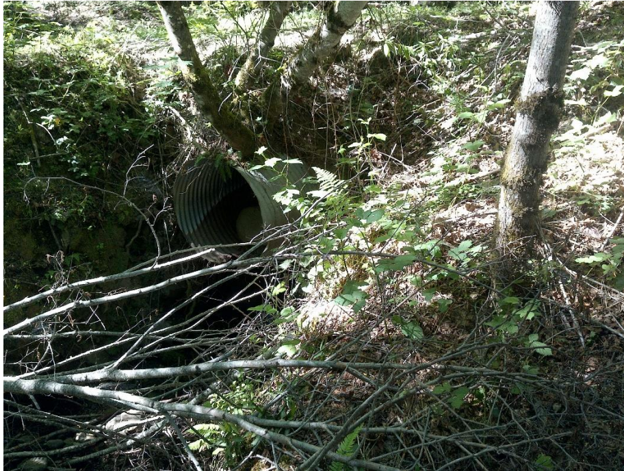
Photo 29— Looking obliquely at the outlet of the 32-inch culvert at WQ 9. The culvert is perched several feet above the channel bed, and the bottom has rusted through.
