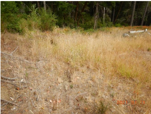
Figure 10. The French drain seems to outlet near the watercourse shown in the distance, just into the trees.
