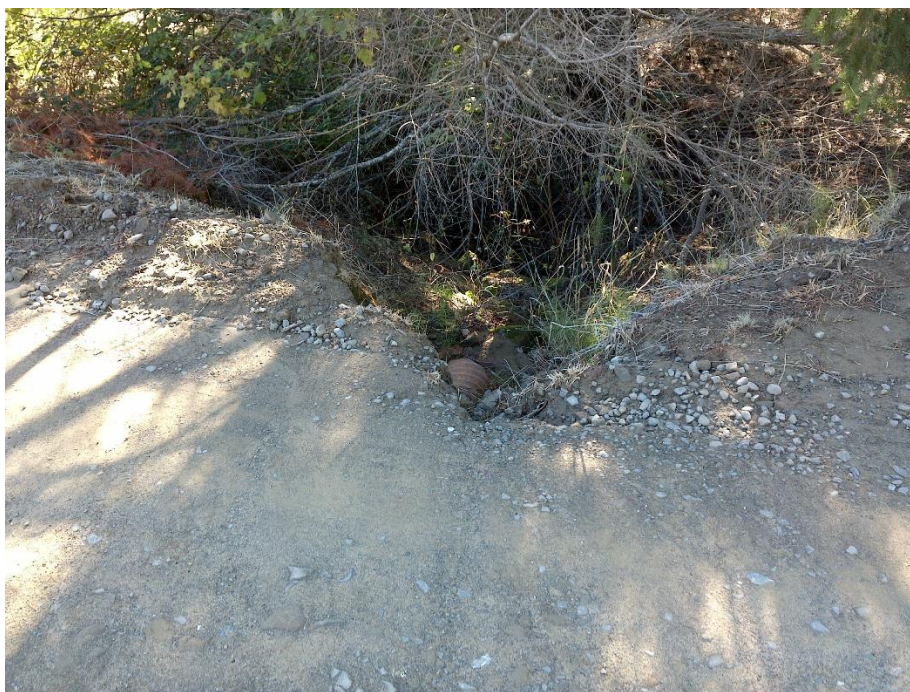
Photo 10—Looking south at culvert outlet at WQ 8. The road prism has failed above the culvert outlet.
