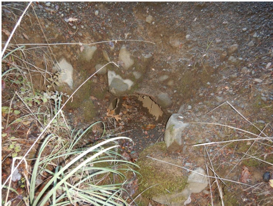
Photo 30—Looking west and downstream at inlet of an 18-inch diameter culvert located at WQ 18.
