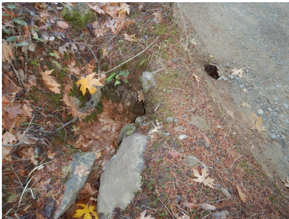
Photo 13—A hole in the road surface connecting to ditch relief culvert below the road located north of WQ 10.
