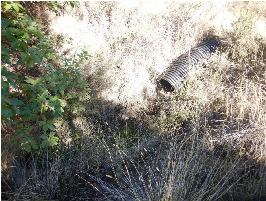
Photo 11—A 24-inch diameter corrugated plastic pipe extending from the road fill at WQ 9.
