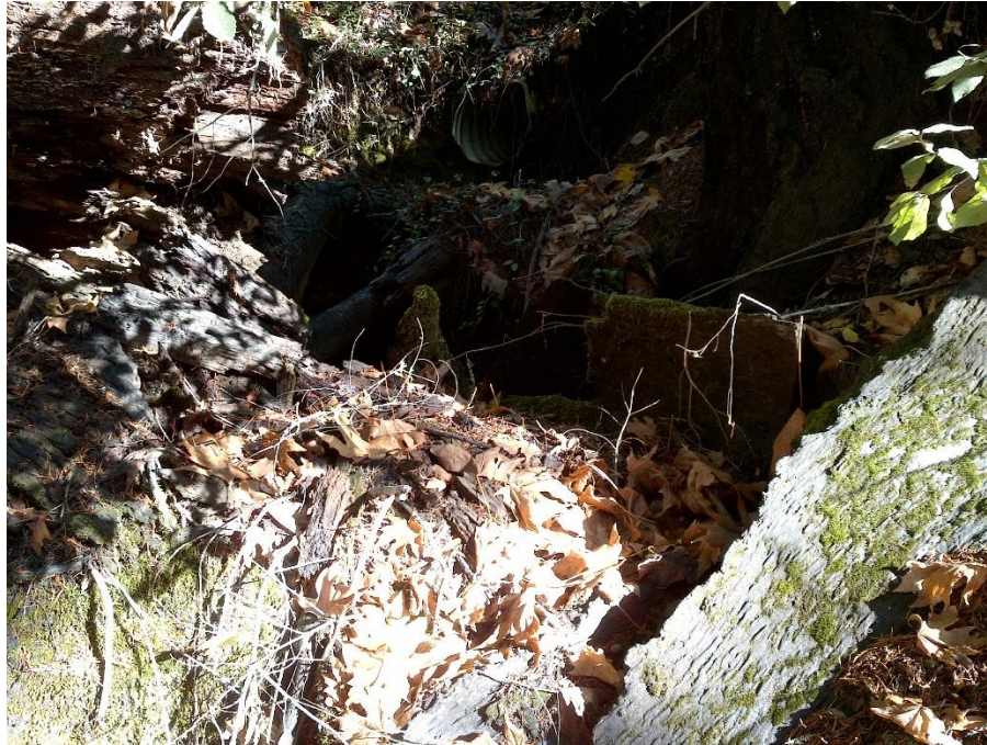
Photo 29—Looking east and upstream at WQ 17 where culvert discharges into the receiving water. The culvert, visible in the top center of the image is perched several feet above the channel.
