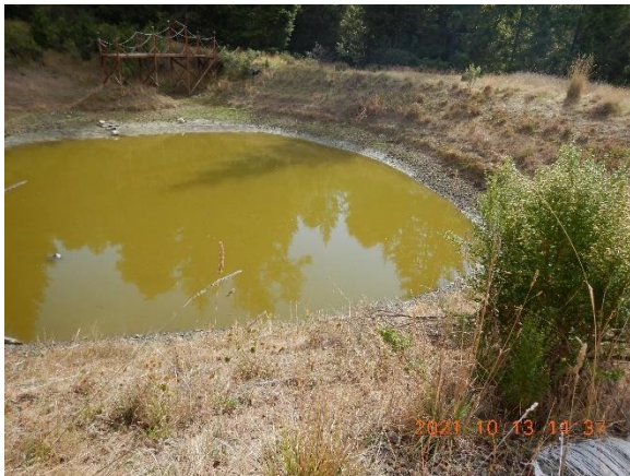
Figure 11. Pond 1 is an unlined pond with earthen berm.
