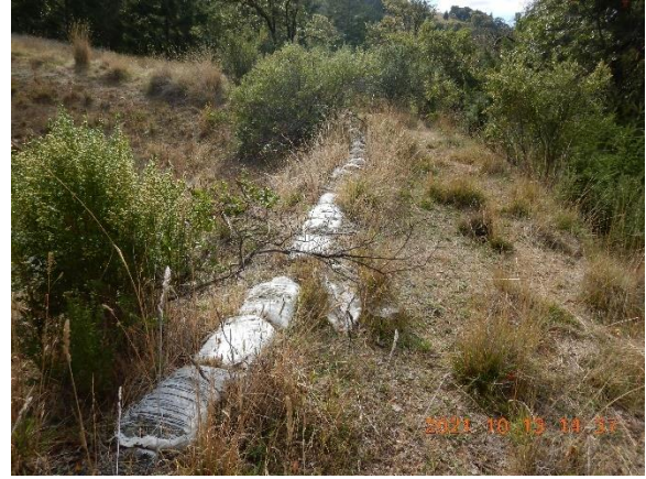
Figure 12. Earthen berm associated with Pond 1 is approximately 12' wide at the top; I did not observe cracks or other indicators of instability.
