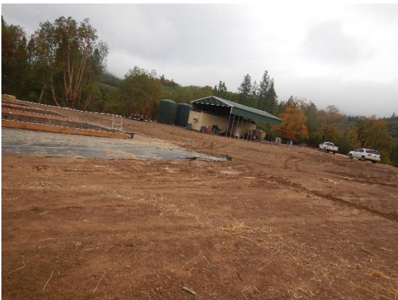
Figure 5. Upper flat looking east. Building has no gutters and the tanks located behind in are at edge of freshly graded flat and are full with water from well.
