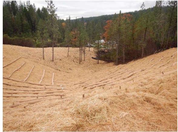
Figure 10. View from top of slope at WQ1. On right top is the location where concentrated water spilled over edge and caused erosion and transport of the recently graded slope material.
