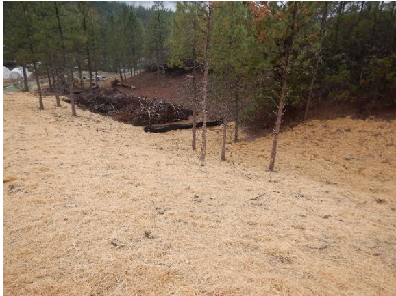
Figure 12. The steep swale levels out; cleared brush piled along the thalweg of the swale remains in place and intercepted sediment being transported and likely helped it settle out. Erosion control measures were applied to that point. Note the silt fence which is shown in next photo.
