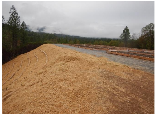
Figure 7. View looking west from top of swale at WQ1, showing from right to left the cultivation beds, the plastic woven fabric underneath, the break in slope, and erosion control measures, including straw and fiber rolls. The slope failure formed a void that now has straw stuffed into and fiber rolls terminate there, leaving the same location vulnerable to reactivation.
