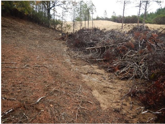
Figure 16. View from swale, looking upslope, with, brush pile, new deposits and natural hillslope. During my inspection, water continued to flow along the surface of this northern margin, on top of the deposits.
