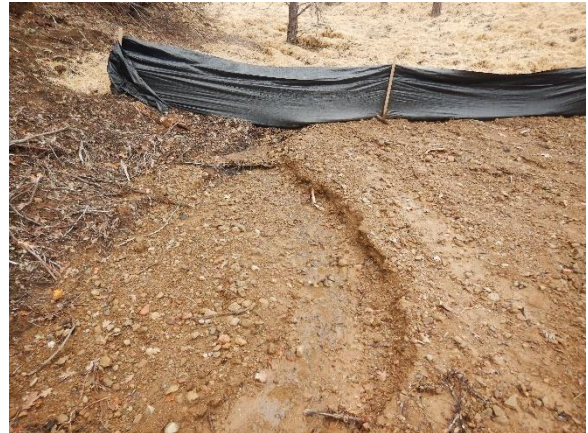
Figure 14. Looking up at the silt fence and settled sediment from the slope failure. Note light color of the fresh deposits.
