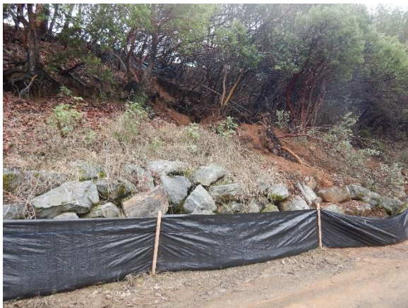
Figure 21. Along the cut bank of the driveway, rip-rap had been placed, according to the landowner prior to his purchase of the Property. Above the riprap is the cleared flat. Runoff from the cleared flat caused fill erosion at the rip rap
