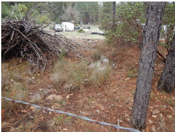
Figure 17. Concentrated water flowed across the parcel line, down a skid road, crosses the ditch on top of culvert and delivers into the neighbors use areas.
