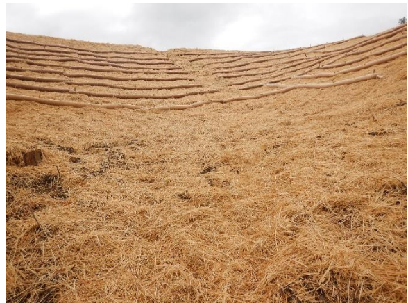
Figure 11. View looking up at slope. The location where the fiber rolls are separated is where concentrated water came down the slope. Straw was pushed in void.
