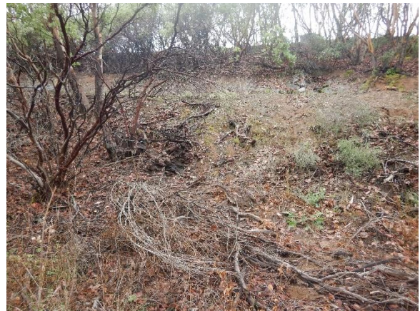
Figure 23. Slope below road at runoff point is sparsely vegetated.
