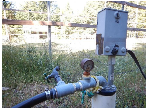
Photo 16: A Closer view of the groundwater well
