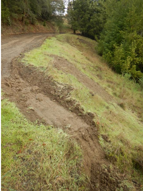
Photo 1, Access Road: Path of concentrated road runoff discharging to hillside
