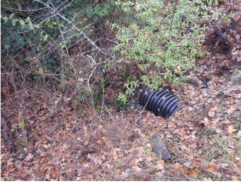
Photo 3, Crossing 3: Outlet of Crossing 3 perched above watercourse
