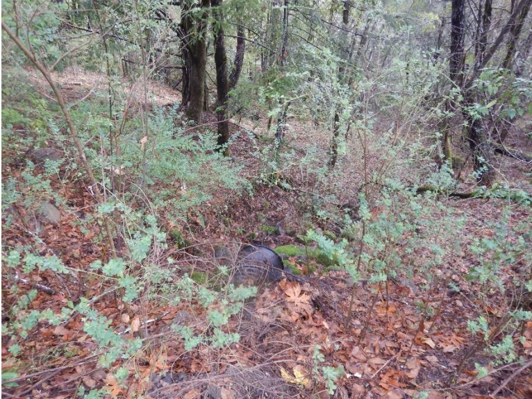
Photo 4, Crossing 5: Outlet of Crossing 5 perched above watercourse
