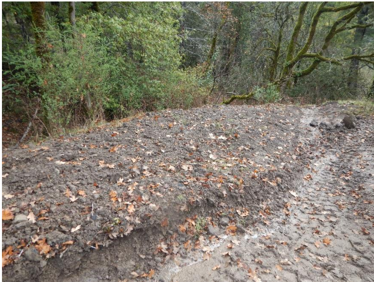
Photo 2, Crossing 2: Road runoff discharging to watercourse near outlet of Crossing 2
