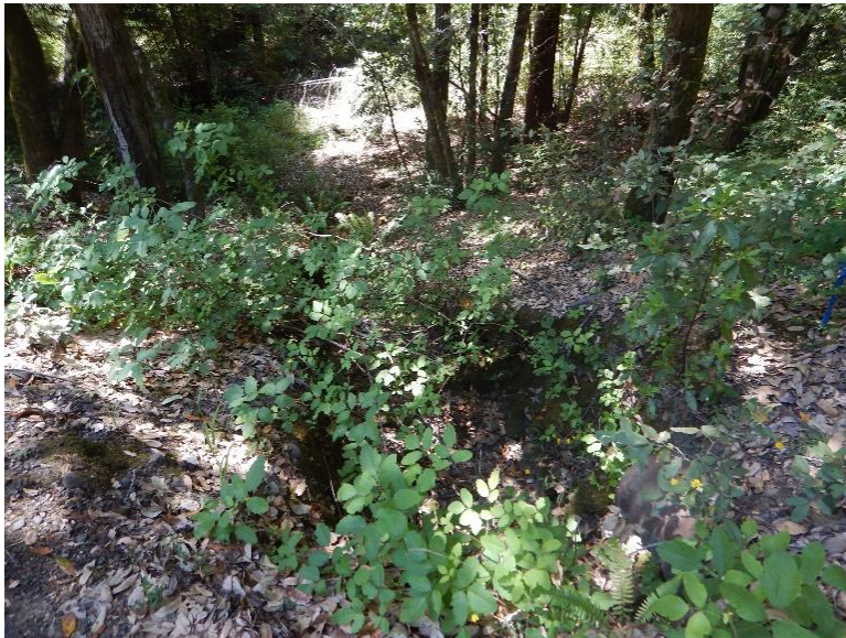
Photo 6: Culvert 3: Watercourse crossing with perched metal culvert outlet
