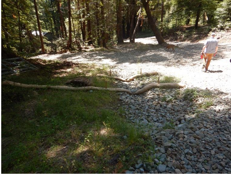
Photo 5: Culvert 2: Rock ford watercourse crossing with freshly installed straw wattles at driveway underlain by buried culvert
