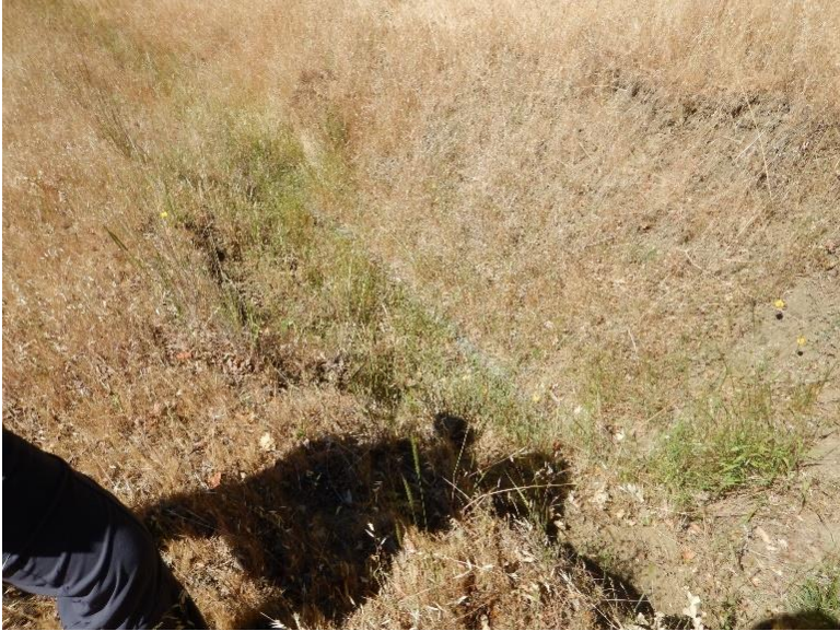
Photo 3: Wetlands Culverts: Partially buried metal culvert in entrenched channel
