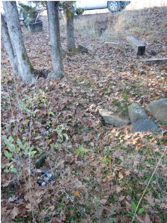
Photo 4, Culverts: Black plastic culvert outlet under access road in background, and black plastic culvert inlet in foreground
