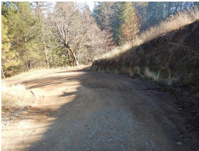
Photo 2, Access Road: Rut across road surface
