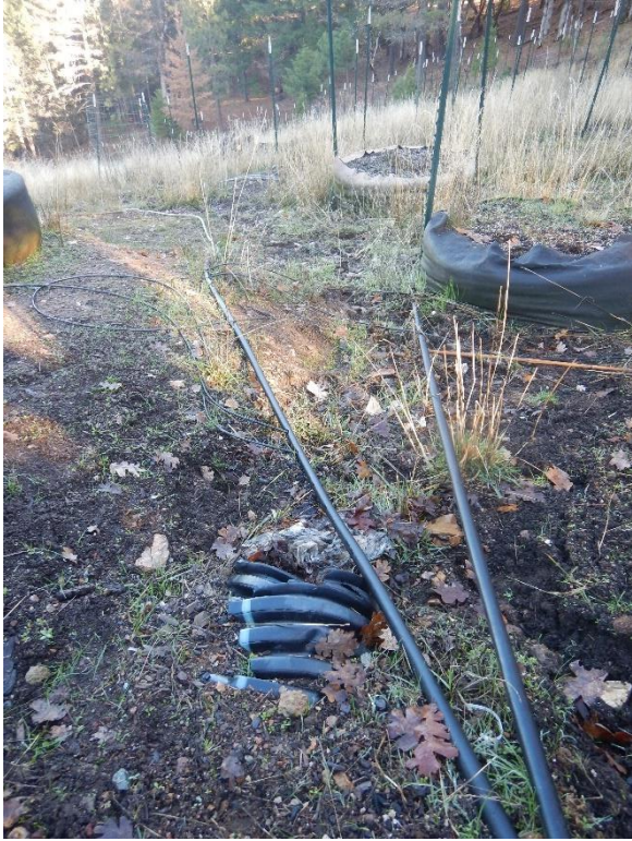
Photo 5, Culvert: Squashed culvert outlet and defined channel below
