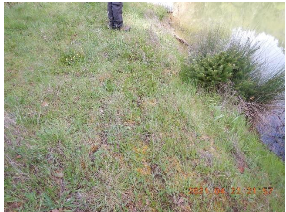
Figure 48. Cracks in berm near outlet pipe.
