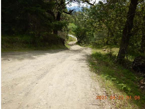
Figure 2. WQ1- steep dirt road segment id located next to watercourse, lacks drainage facilities or surfacing, and has developed rills and threatens sediment delivery to watercourse.
