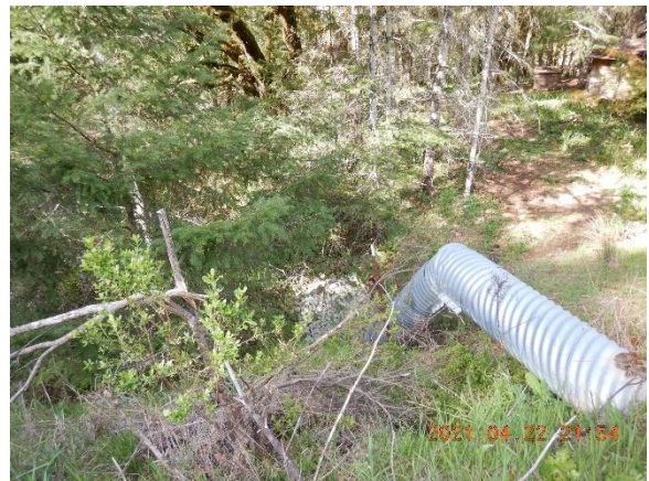
Figure 49. Pond outlet pipe downspout to channel with rock recently placed.
