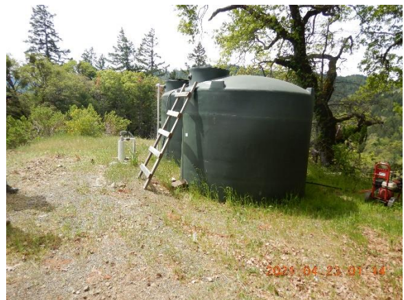
Figure 42. Well and water tanks at 486.
