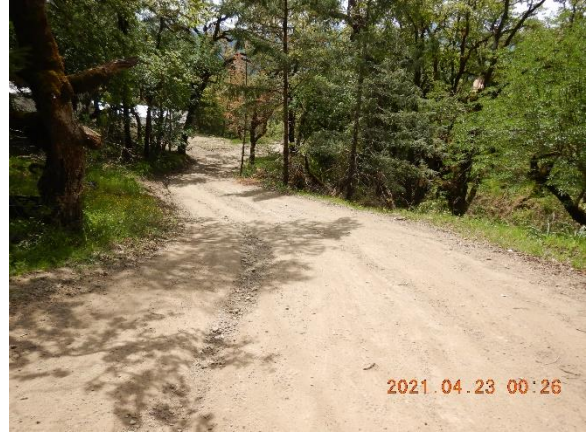
Figure 20. Riparian road at WQ6 lacks drainage structures and is hydrologically connected to adjacent watercourse.
