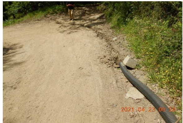
Figure 25. A drain pipe from the greenhouse at WQ7 is discharged on to the road near 484.
