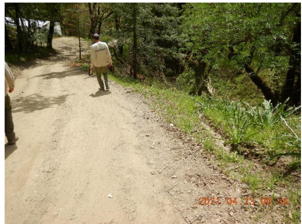
Figure 21. Discharge from road to steep slope to watercourse.
