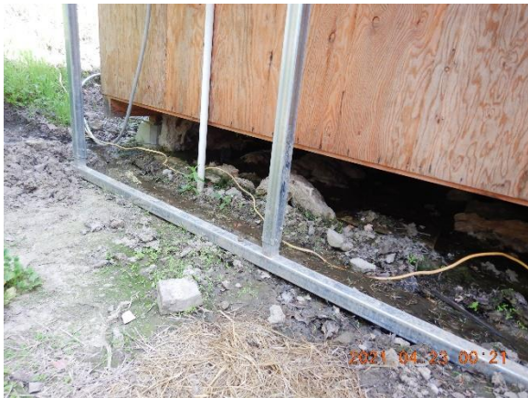
Figure 19. A daylighted seep located along a cut bank is ditched and routed around the building and discharged to the hydrologically connected road at WQ6.
