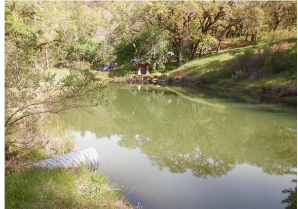
Figure 47. Pond at overflow pipe, minimal free-board.
