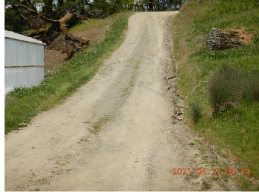
Figure 15. Rills on hydrologically connected steep road segment.
