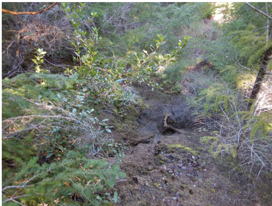
Photo 11—Significant erosion of the northwestern corner of the Glass House pad from stormwater concentrated by the Glass House pad. Panther Canyon is in the background of the image.
