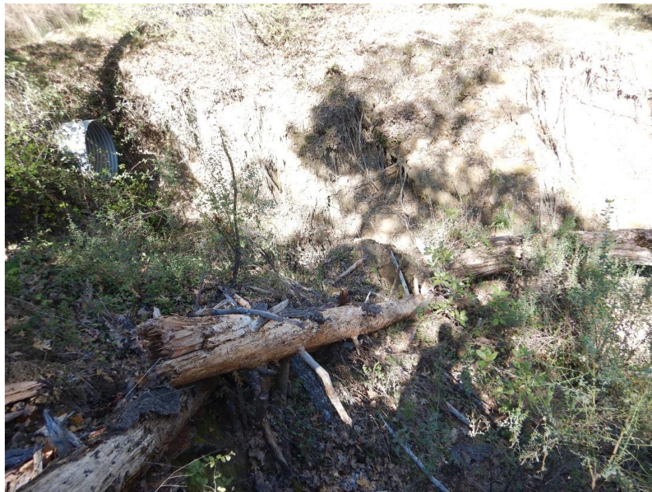
Photo 20—Looking north at culvert outlet at RP 84. The culvert is perched several feet above the channel bottom and directed at the unarmored left bank of the watercourse.
