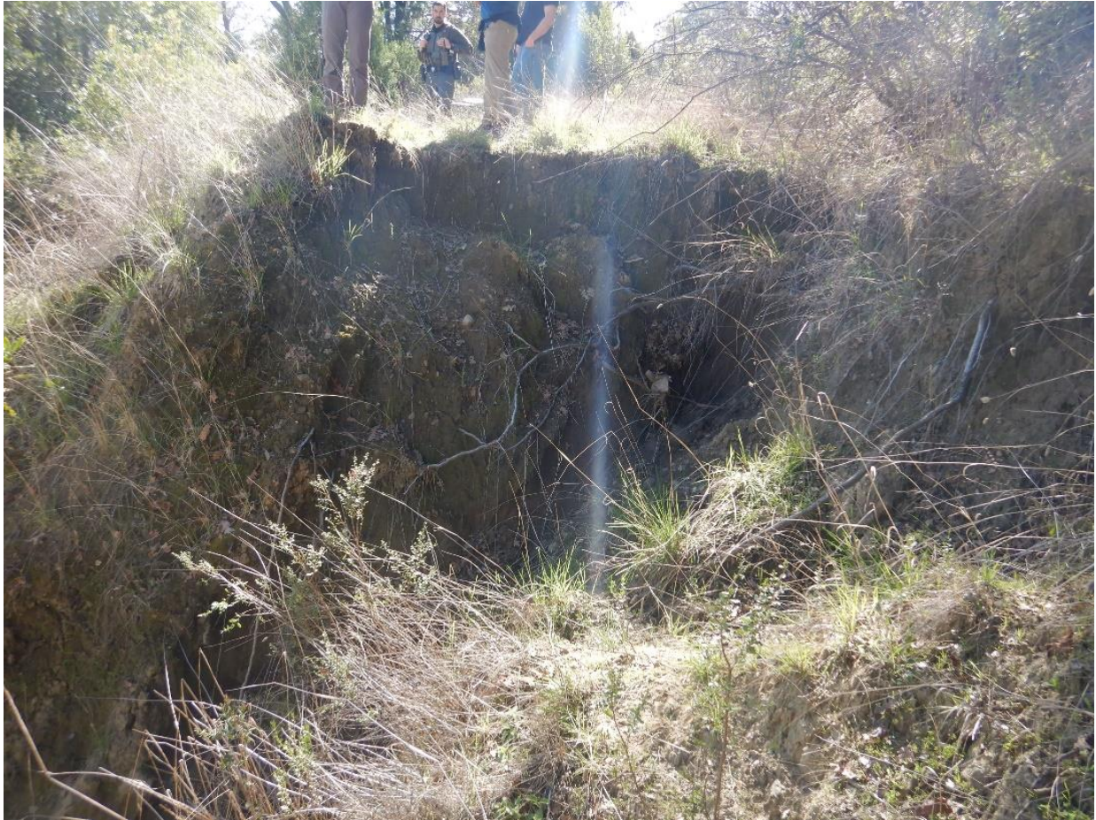
Photo 23— Looking south at a failed road crossing on the unused road east of Shady Grove.
