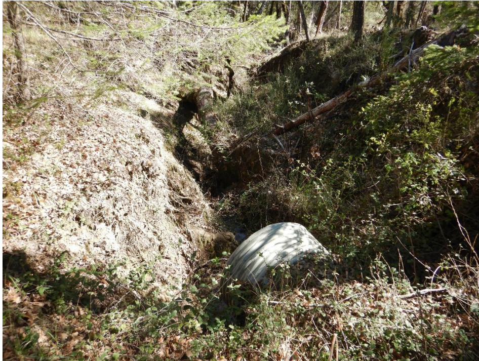
Photo 21—Looking east and downstream at the same culvert in the previous image.
