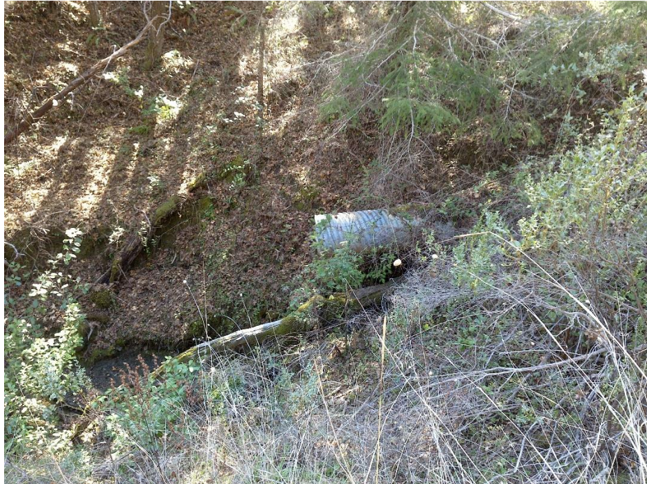
Photo 22—Looking south at a perched culvert on the unused road east of Shady Grove.
