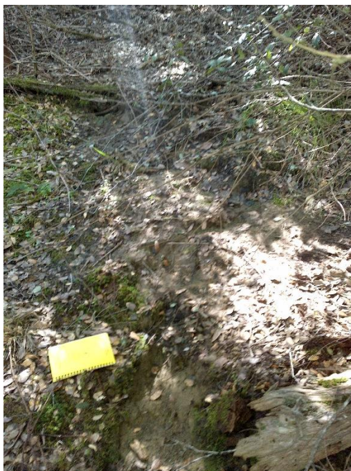
Photo 10—Scouring immediately downslope from the single gutter outlet discharging stormwater collected by the Glass House's roof at the northwestern corner of the Glass House.
