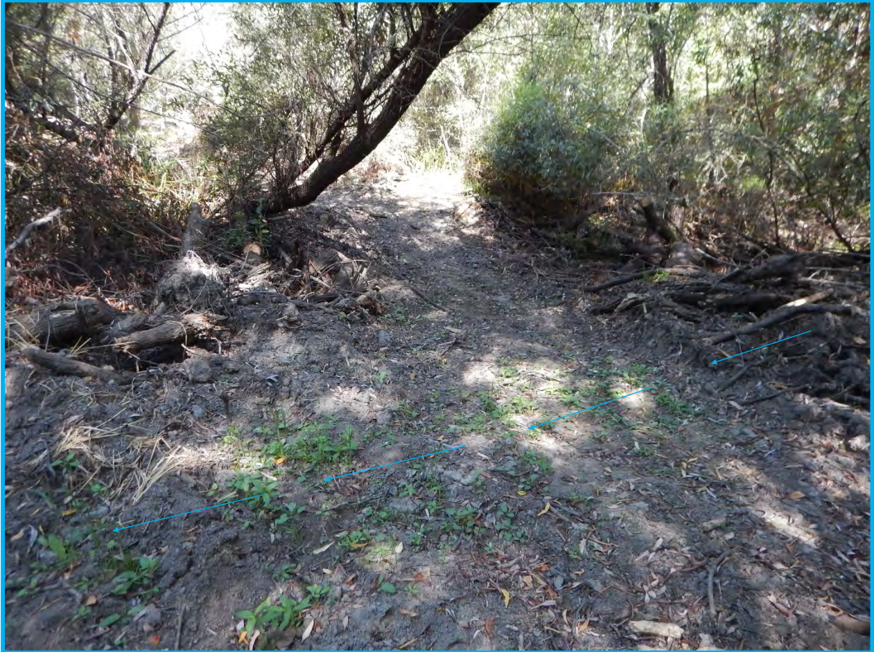
Photograph 8. The road crossed a major overflow channel as it headed towards Atascadero Creek. Riparian trees were felled using chainsaws and heavy equipment pushed the fallen trees into the riparian forest. Fill consisting of fallen and cut trees, understory vegetation, and soil had been placed in the overflow channel. Blue arrows show flow direction during high water.
