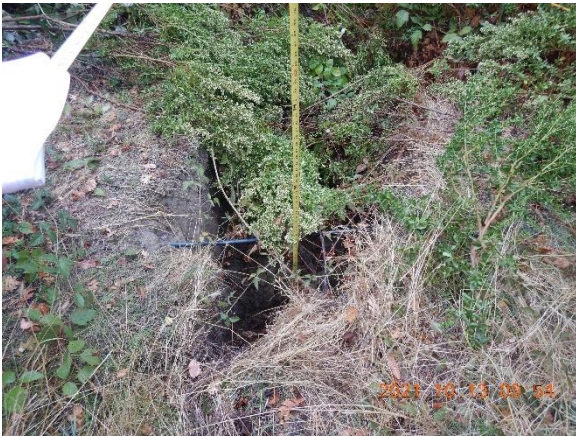
Figure 13. Gully at outboard edge of roadway at WQ1, at WP610.
