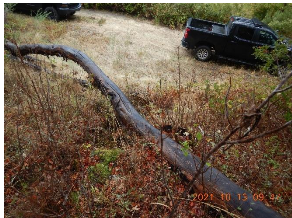
Figure 11. As watercourse hits cut bank, it has eroded a gully at WP 608. The road is constructed across the watercourse, with no conveyance structure.
