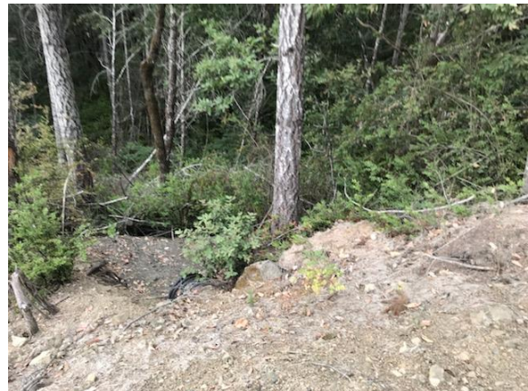
Figure 7. WQ3 - DRC outlet; it should be monitored to ensure no sediment delivery to the watercourse.
