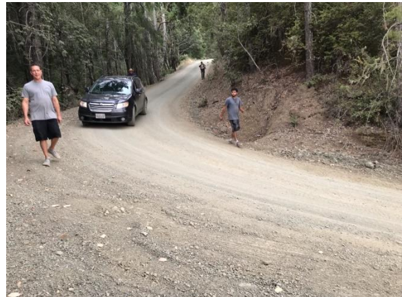
Figure 6. WQ3 - The road segment below the first terrace is steep and adjacent to the Class II watercourse, and appears to be within the 100' Class II setback of the watercourse. The road could use shaping to ensure that water goes into the ditch relief culvert.
