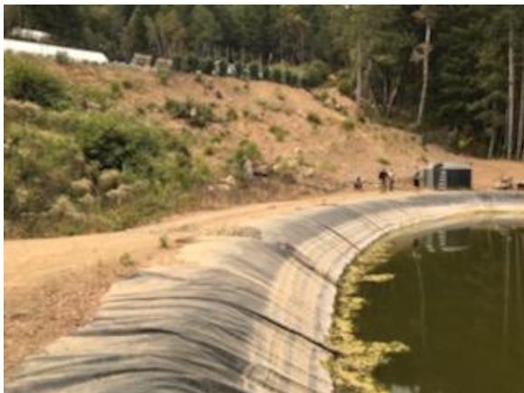
Figure 18. View of slope above pond. There are stumps in the slope, indicating natural ground.
