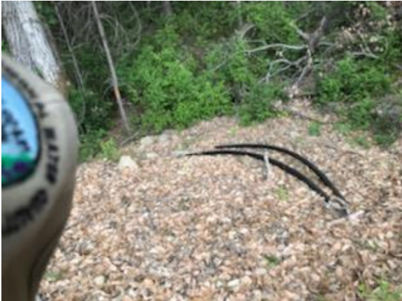
Figure 21. Flexipipes associated with cisterns draining pond from beneath liner. They are placed in the fillslope of the lower flat, below the outboard edge of the road, and discharged on to the ground surface, toward the Class II watercourse, downstream of Crossing 2. There is no armoring.
