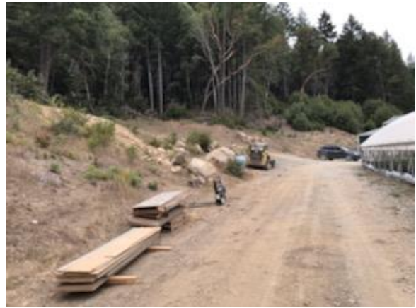
Figure 10. Outlet of DRC is the middle cultivation area and without outlet protection.
