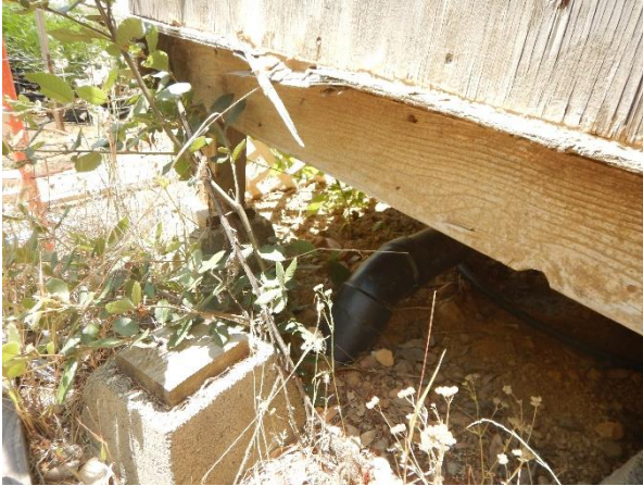
Photo 7: View of assumed septic related piping at the residence.
