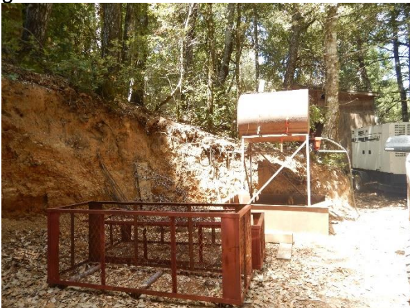
Photo 11: Above ground storage tank and generator located below the water tank.
