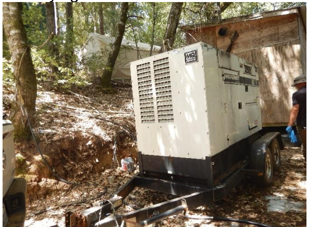
Photo 12: Closer view of the generator and drying shed behind.
