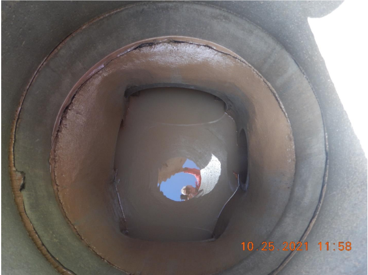
Photo 27: Pondered turbid storm water observed in the bottom of a storm drain manhole.
