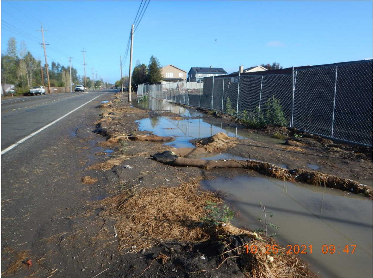
Photo 22: Looking north on Stony Point Road along the project boundary. Roadside wattles on Stony Point Road are destroyed.
