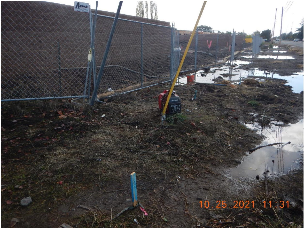
Photo 29: A small generator and water pump in the orange perforated bucket was pumping roadside pooling stormwater back into the Project site.
