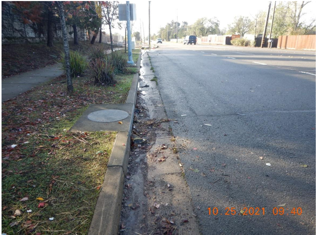
Photo 12: Looking south at the municipal storm drain inlet on Stony Point Road (Map 1). As originally observed during the October 23, 2021 inspection, the storm drain inlet is still obstructed by a weighted wattle and debris. The obstruction at this storm drain inlet contributed to the flooding observed during yesterday's rain event.
