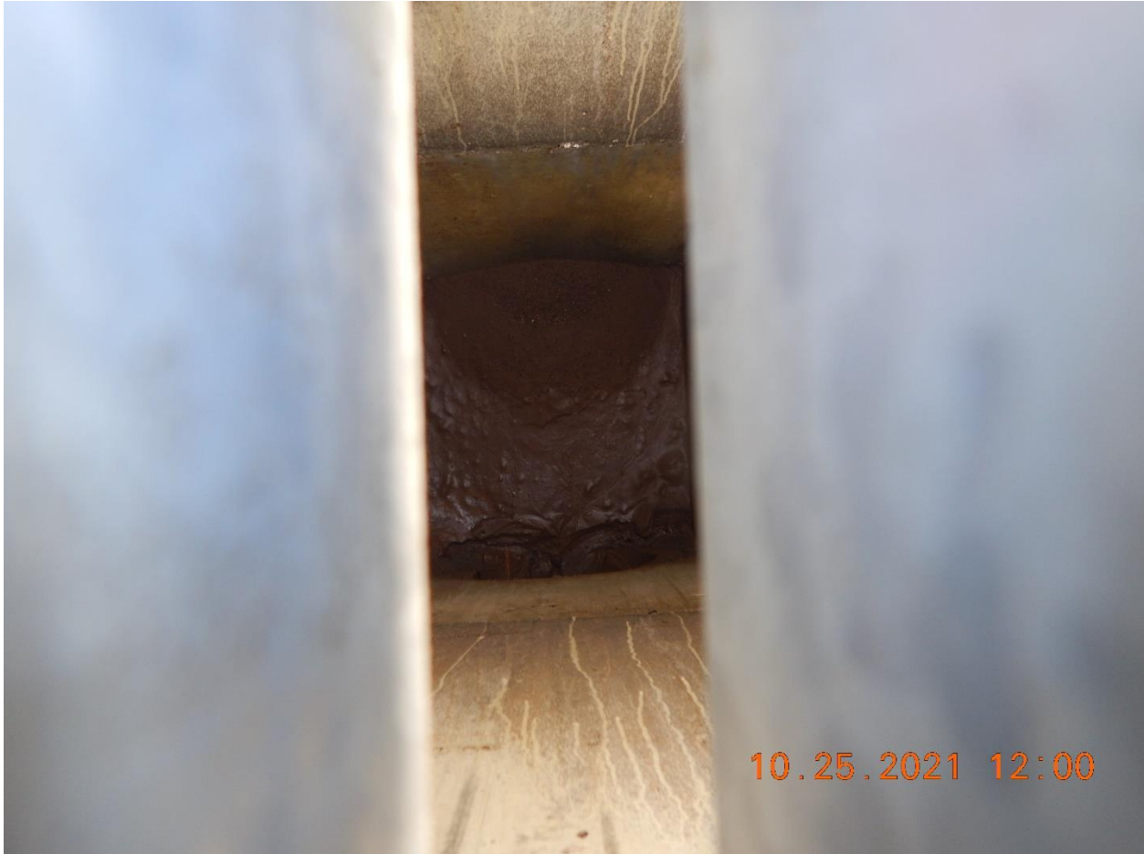
Photo 28: View inside another drain inlet with a grate cover. Sediment deposition is visible, but there is no pooled water visible here.
