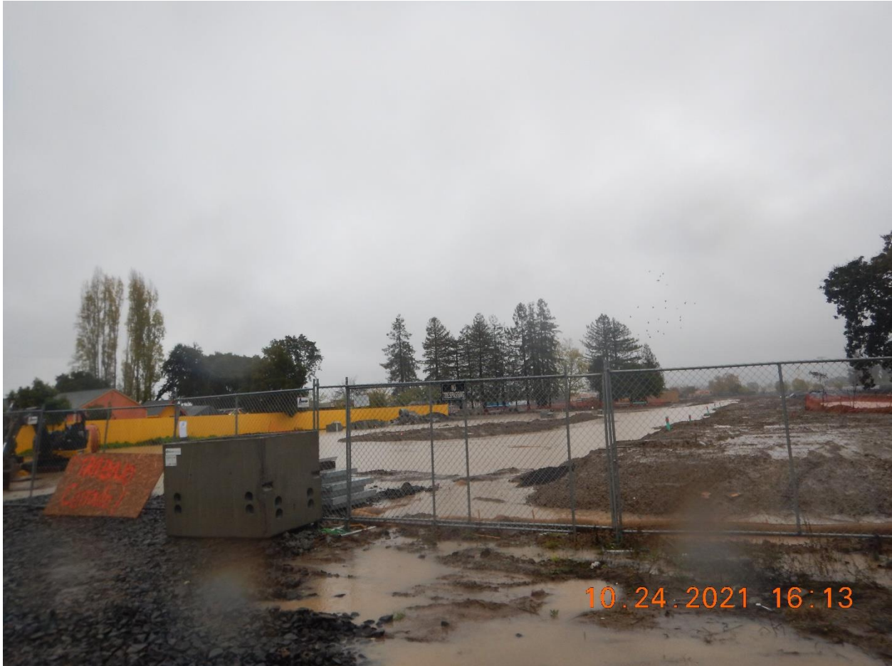
Photo 10: The Southern Entrance of the Project (Map 1), viewed from Stony Point Road. Turbid waters are ponded throughout the site and flowing toward Stony Point Road. The wattle along the fence line is staked, but not trenched in. Also, the disturbed soils on both sides of the wattle are unprotected. Erosional rills are visible on the slope of the earthen pad.
