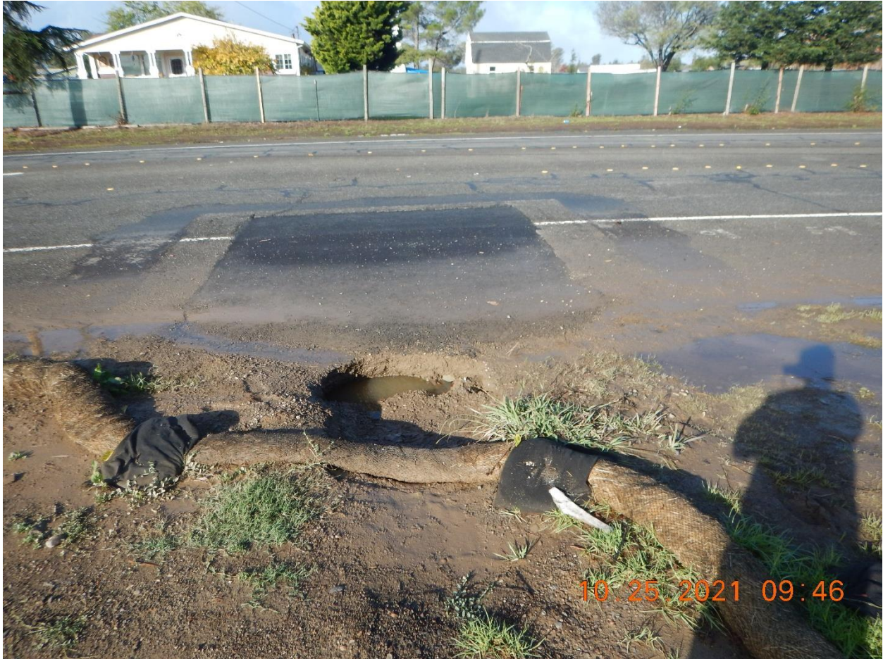
Photo 18: Another location with an asphalt patch, similar to that shown in Photo 17. I could see water trickling into the hole(s) near this patch, which is along the Project boundary on Stony Point Road.
