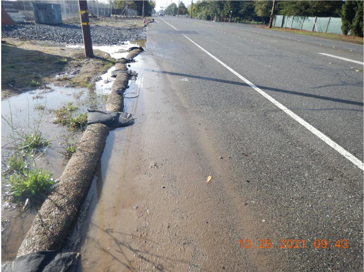
Photo 16: The rocked Southern Entrance of the Project. Sediment deposition is visible beyond the straw wattles on the asphalt of the public roadway, deposited thickly enough that such that my footprints can be distinguished.
