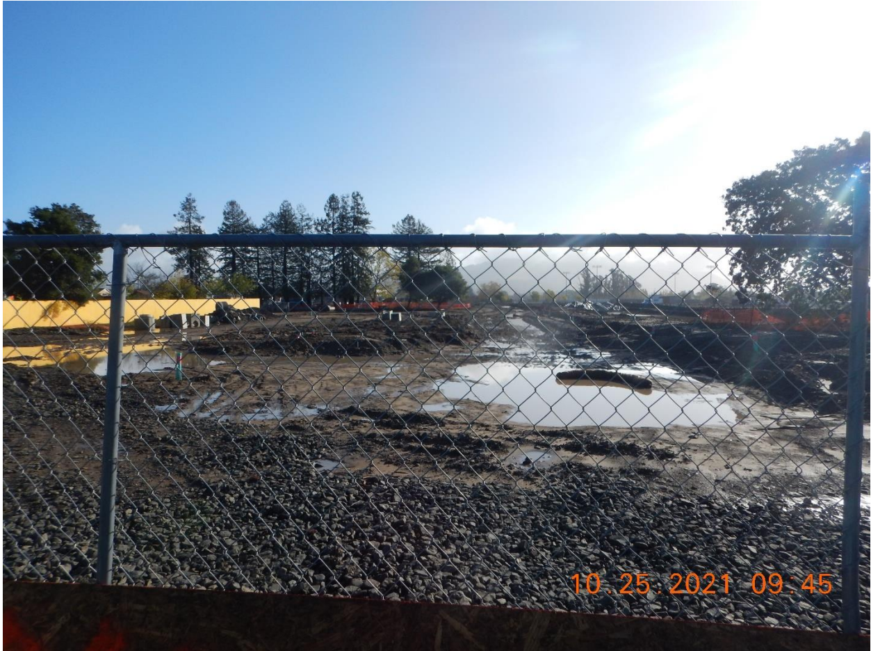
Photo 21: Looking east from Stony Point Road near the South Entrance of the Project. The road system, referenced in Photo 20 above and also observed completely full during yesterday afternoon's (October 24, 2021) rain event inspection is now nearly drained.
