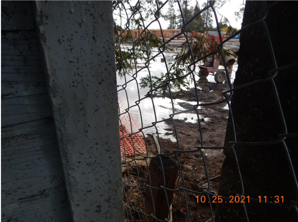
Photo 30: Discharge hose extending from the small generator and pump system shown in Photo 29. The ponding water near Stony Point road was being directed towards an earthen pad within the Project boundary.
