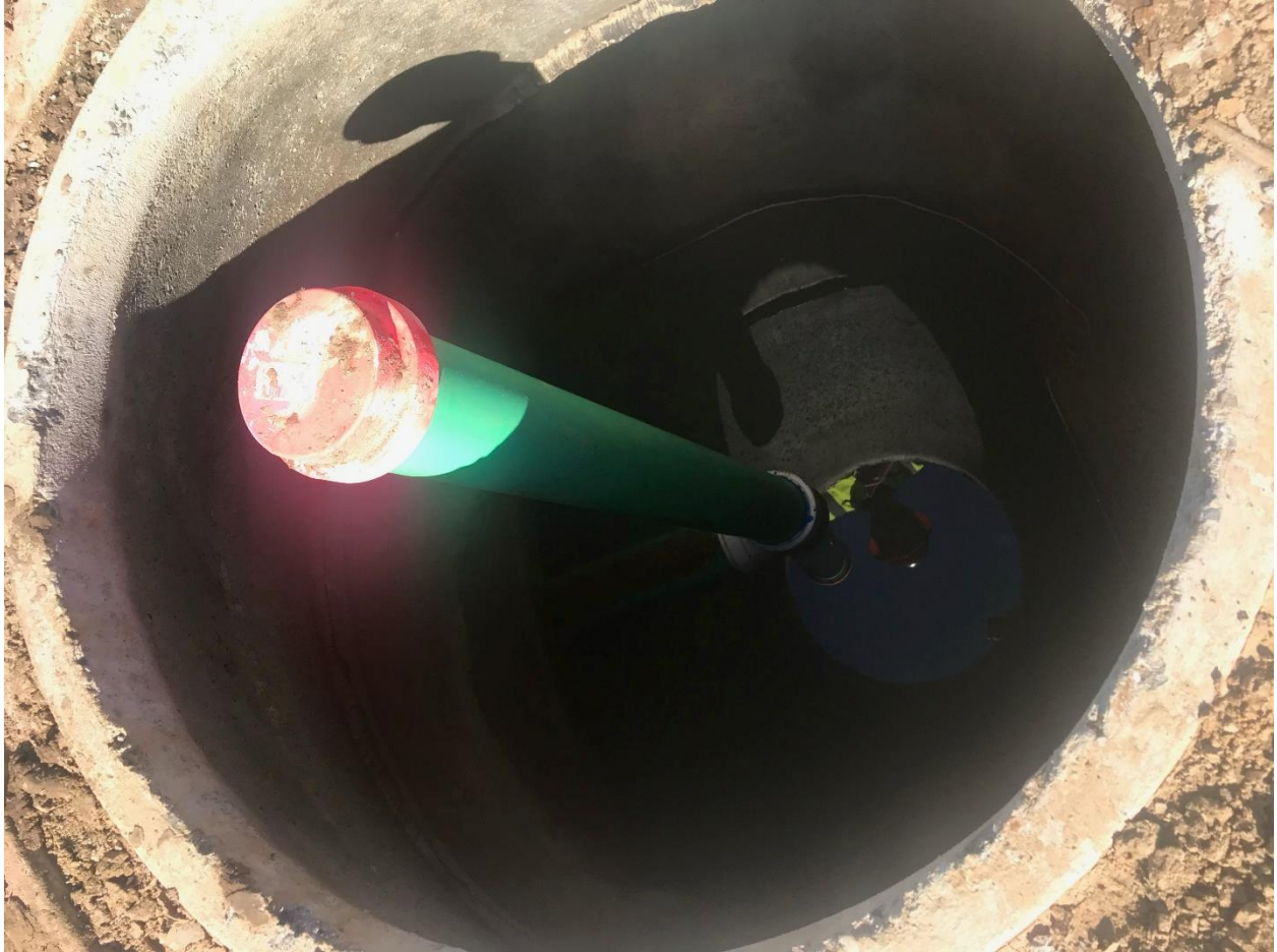
Photo 32: New 4-inch riser pipe and cap installed on previously uncapped 4-inch bypass pipe within a manhole on Site (referenced in Map 1 as either Municipal Storm Drain: North Connection or South Con). Note the sediment deposition on the horizontal pipe that does not continue over the white 90 degree joint. This provides evidence that the vertical pipe and cap was not plugged in this manner during the last rain event. The 4-inch pipe leads to the City of Santa Rosa's public storm drain system. Note the sediment deposition on top of the 4-inch pipe and the pooling water near the bottom rim of the 4-inch pipe. (Photo provided by City staff Nick Sudano on November 8, 2021. Photo taken by City staff Javier Fernandez on October 29, 2021 as documentation that the pipe had been capped).
