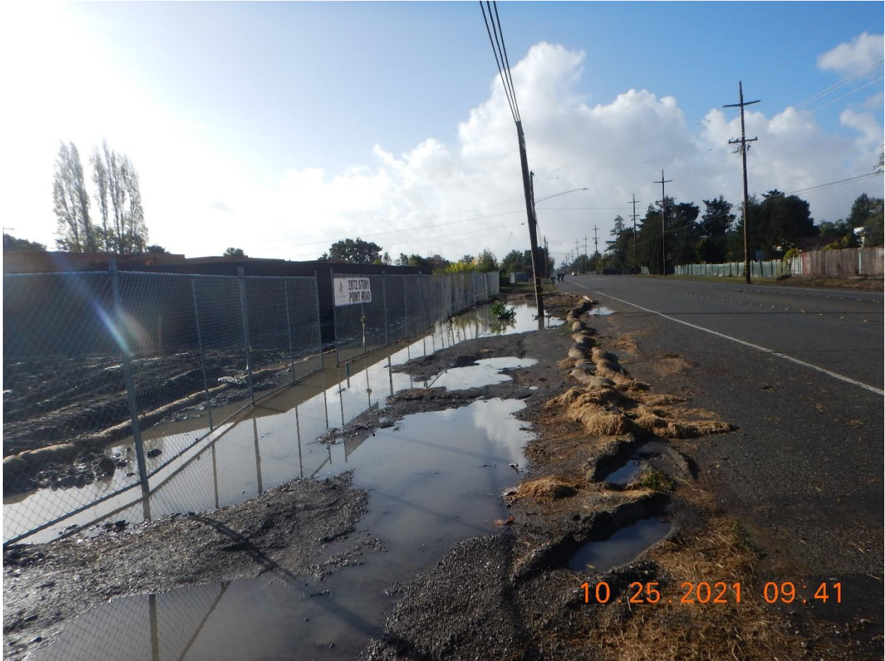
Photo 14: Roadside wattles along the road near the Site's North Entrance are deteriorating. Note that the disturbed soils to the left of the wattles are relatively unprotected and, at a minimum, partially drain towards the public roadway system.
