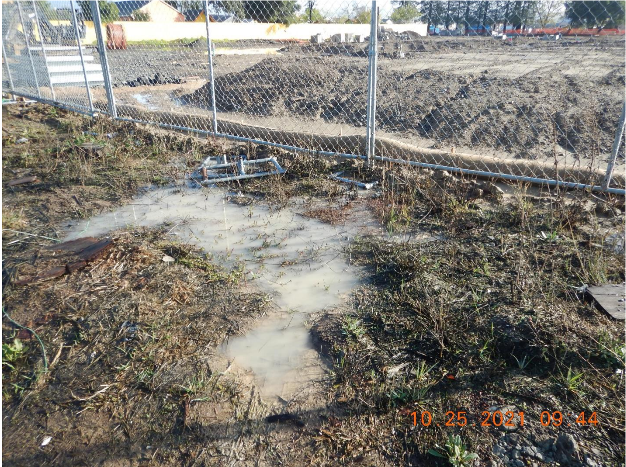
Photo 19: Evidence of erosion on the pad slope, near the South Entrance. Note the rills and sediment deposition immediately behind the wattle, with turbid waters leading beyond the wattle and immediately towards Stony Point Road.
