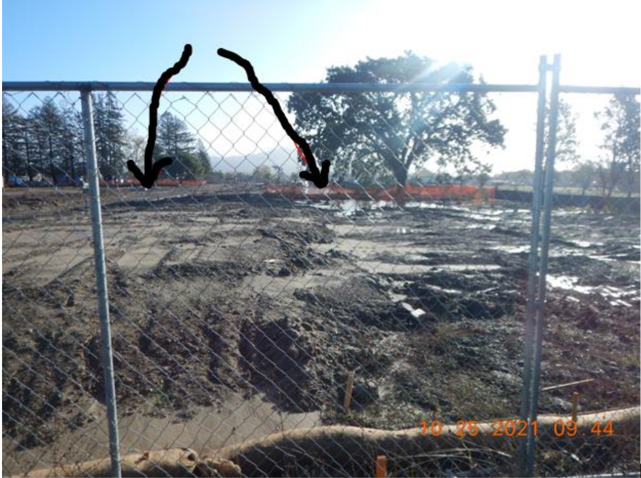
Photo 20: Looking East from Stony Point Road near the Southern Entrance of the Project. The left black arrow indicates the location of the rough graded future road system which is now almost completely drained of ponded water. As noted above, I observed during my inspection the previous day (October 24, 2021) that this road system was completely full of water. The black arrow on the right indicates the South Ponding Area, with significant ponding still present. The area on the right appears to be retaining the water, while the area on the left appears to be drained.
