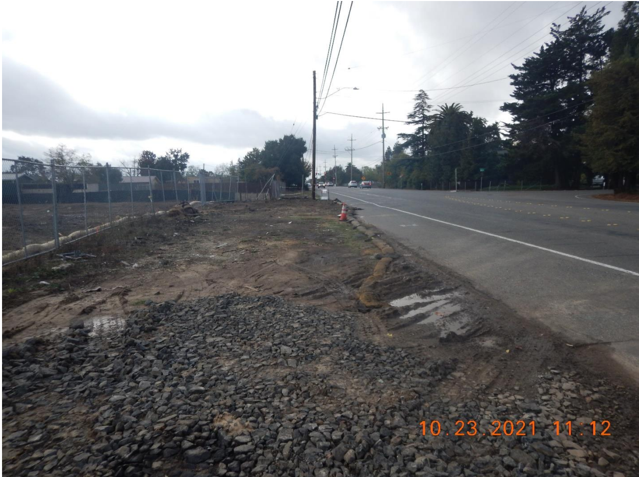
Photo 3: Looking south from near the South Entrance, the disturbed area continued beyond the metal chain link fence on the left to the edge of Stony Point Road on the right. The two linear sets of roadside wattles are partially destroyed, and the fence line wattle is not trenched in. The South Entrance had a rocked entry way to the gate, which is evident in the foreground.
