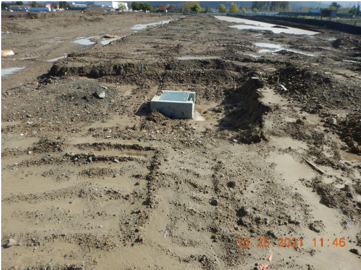
Photo 24: Looking east within the Project near the south boundary. Note the storm drain and future road system with little to no standing water and compare it to the pooling area to the right. The water pooling on the right is also shown in Photo 25 below. No minimum erosion or sediment control BMPs are present on the Site and the storm drain inlet is unprotected.
