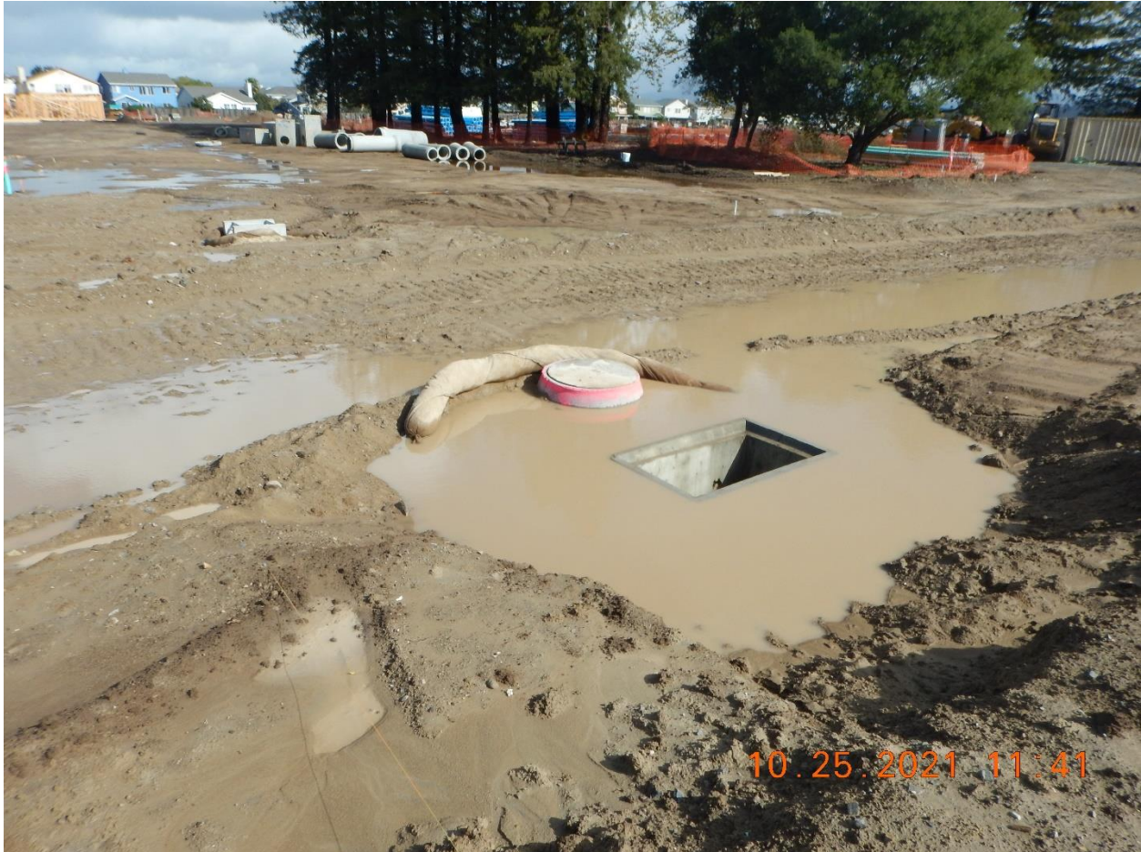
Photo 26: Pondered storm water around a storm drain inlet. The pondered water is at the exact level of the top of the concrete inlet but there is no water inside the drain inlet at this time. If the downstream storm drain system were plugged, one would expect that this storm drain inlet would be completely full to the same level as the pondered water observed around the inlet. The single wattle is the only BMP seen in this area and is completely ineffective.
