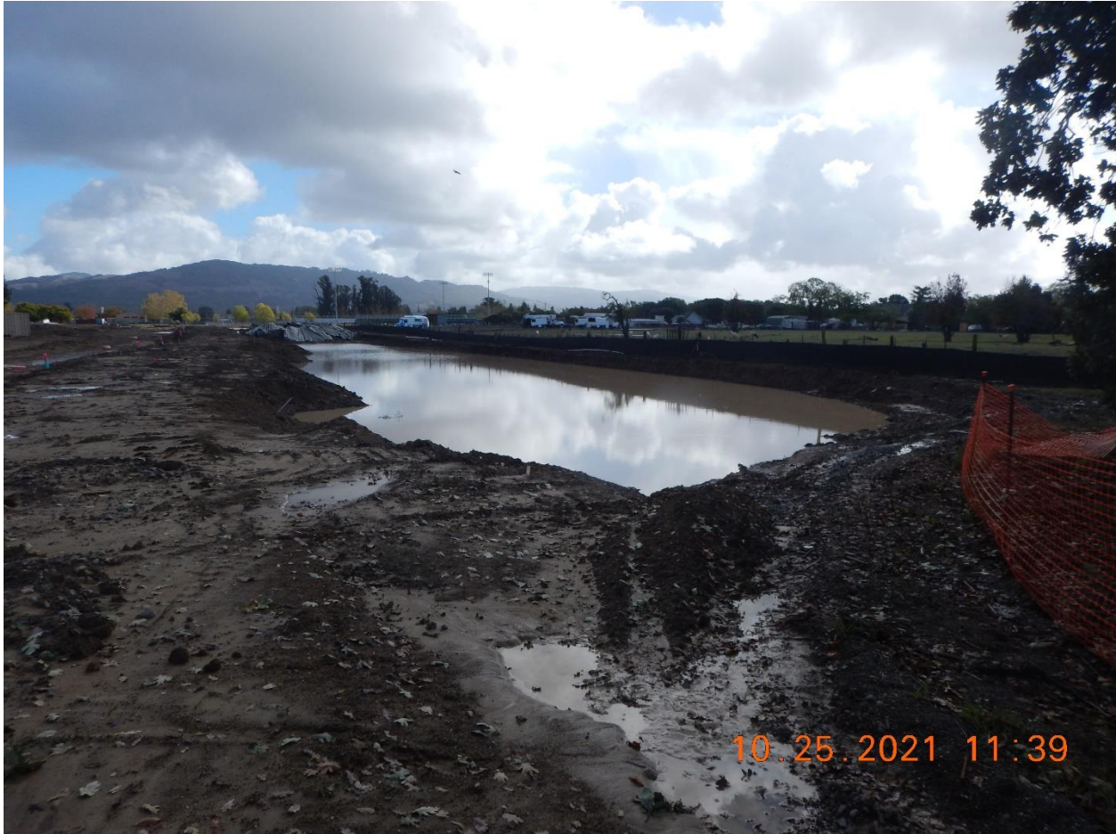
Photo 25: Photo of the area I refer to as the South Ponding Area in this report. This feature is not connected to the rough graded roadway system and storm drain system, and there is still significant water impounded in this area. No minimum erosion or sediment control BMPs are present.
