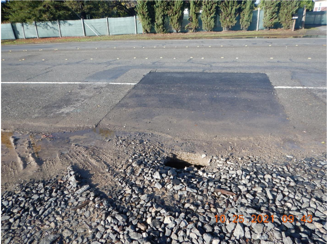
Photo 17: One of the square asphalt patches I observed along the project boundary on Stony Point Road. I observed water trickling into the holes near these patches.
