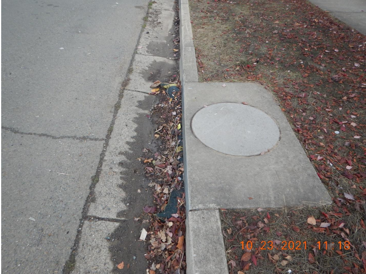
Photo 4: I observed a City of Santa Rosa Municipal Storm Drain Inlet along Stony Point Road, near the North Entrance (Map 1). Note that the inlet is nearly plugged with a weighted wattle and debris.
